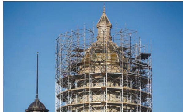
The Capitol Square Project is on track to be finished next year. Jacob Byk/Wyoming Tribune Eagle
