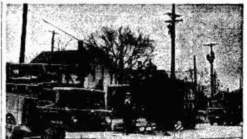
PORTABLE TRANSFORMER READY . . . The Northern States Power Co. installed two powerful portable transformers on its main line on Chestnut Street leading to the plant. Should the dike break, putting the
