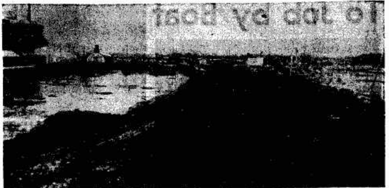
DIKE PACKER . . . A diesel crawler tractor compacts dike along Crooked Slough as work nears completion. View is to the west. Water at left is seepage pool forming in adjacent rail yards. (Sunday News photo)
