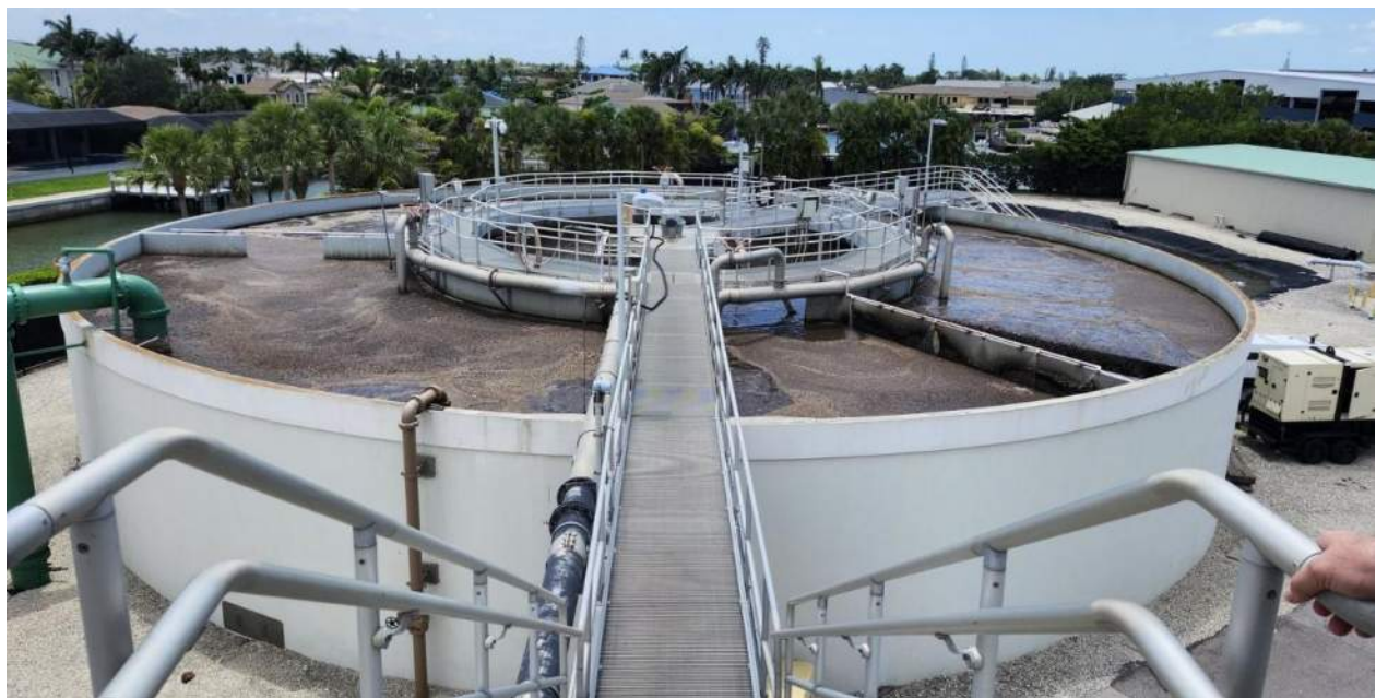
Figure 3-1 Existing MLE Tanks
