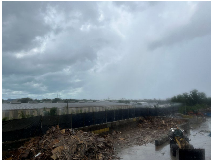
Figure 3: NW view of misters on West Perimeter fencing
