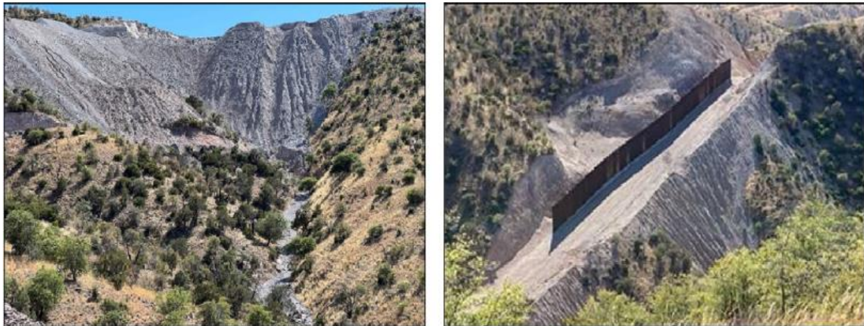
Erosion below the site of a cleared staging area (left); erosion below an area where only several border barrier panels were installed as of January 2021 (right).
