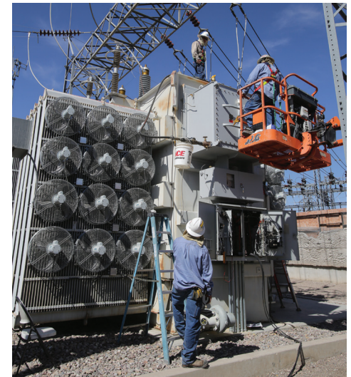
TEP employees install upgrades at the East Loop substation. The planned transmission line would connect East Loop to new and existing substations.
