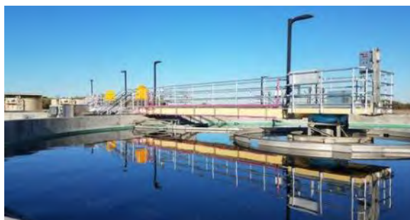
Marana Wastewater facility. Source: Town of Marana
