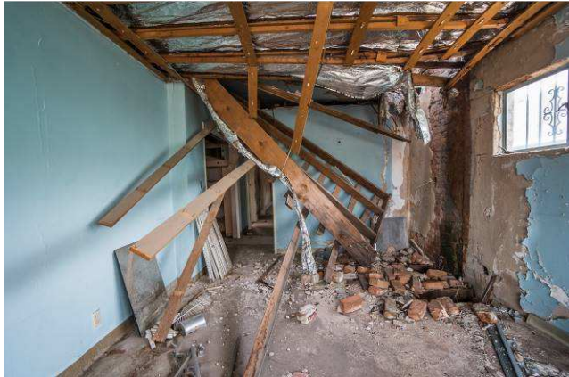
Collapsed beam and ceiling
