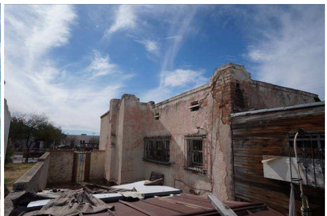
Missing Stucco at chimney, weather-beaten windows
