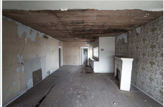
Plaster ceiling damage
