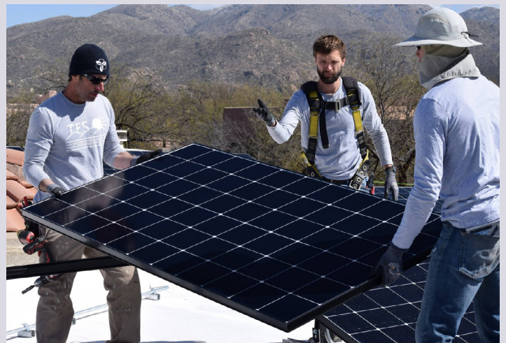
↑ Photo courtesy of Technicians for Sustainability
