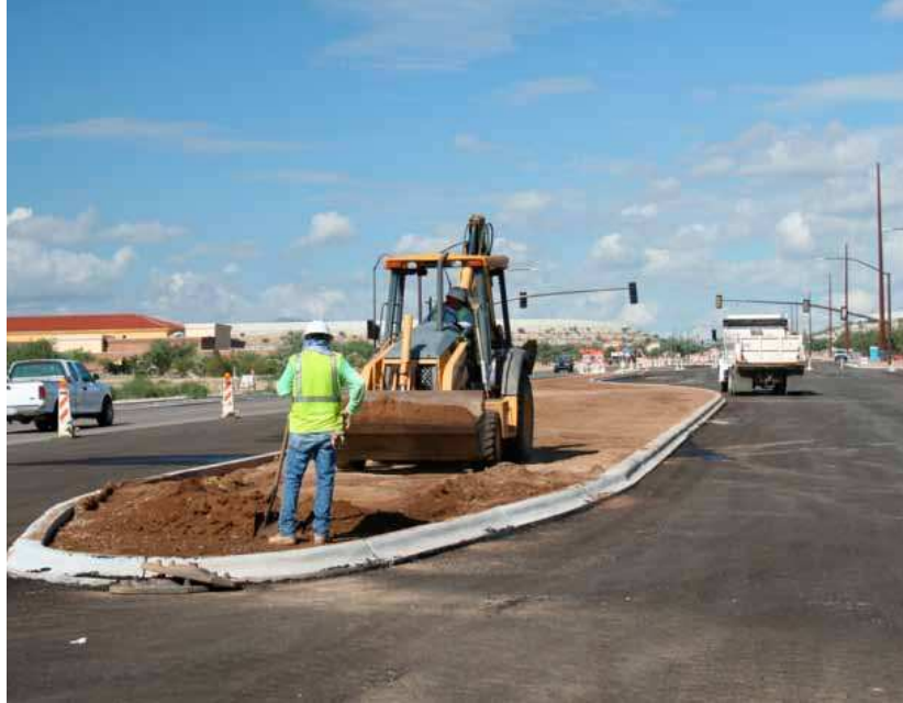
Building a raised median as part of the La Cañada improvement project.
