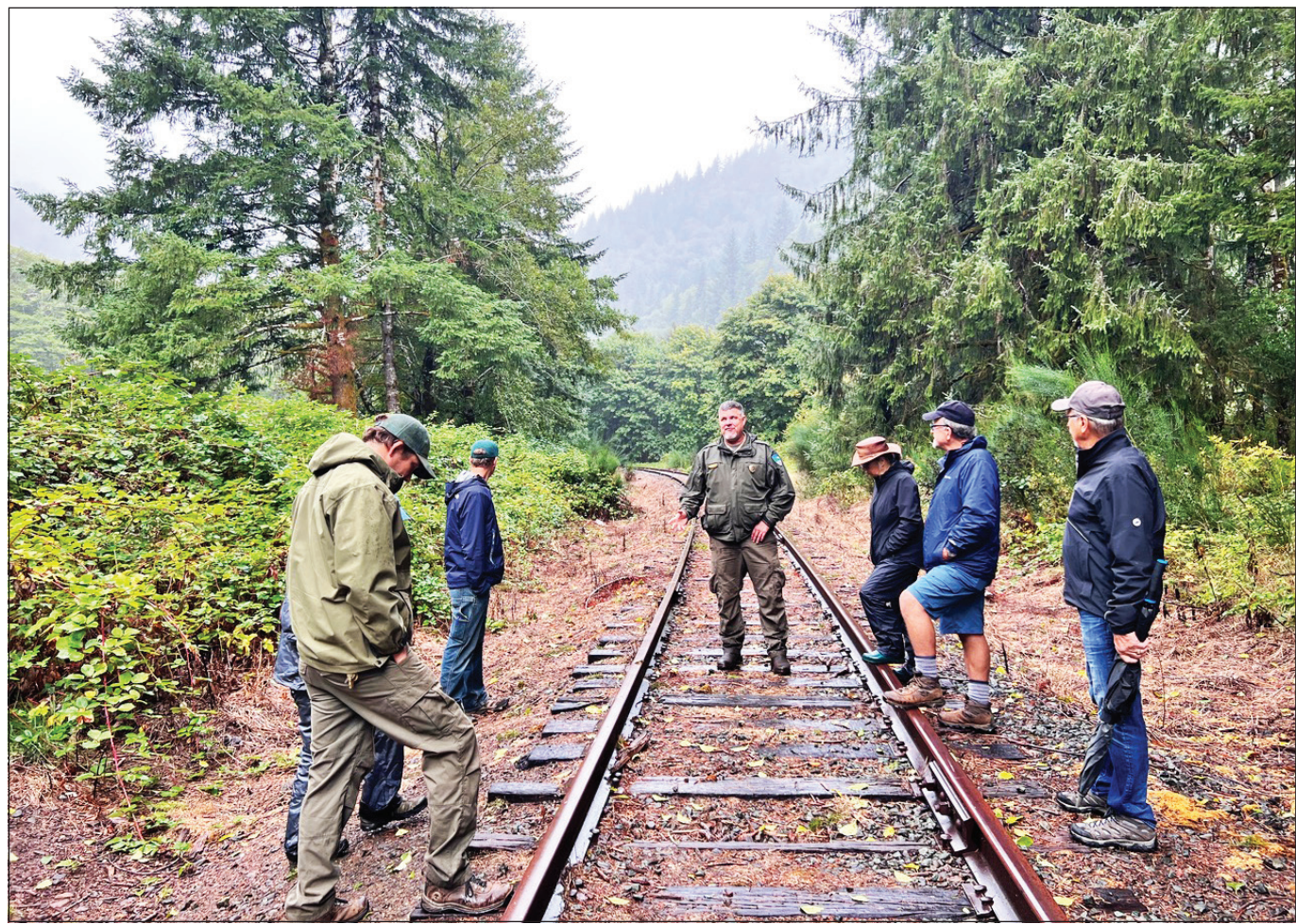
Members of the Salmonberry Trail Intergovernmental Agency board visiting a portion of rail in Cooper Valley with an Oregon Parks and Recreation Department official prior to the meeting in Wheeler. PHOTO COURTESY OF THE SALMONBERRY TRAIL FOUNDATION
