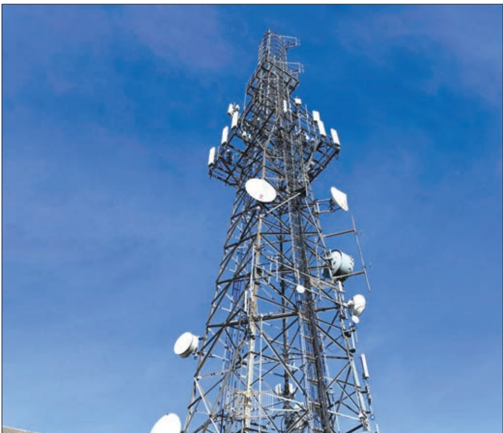
One of the twelve radio towers, atop Mount Maxwell, that make up the county’s current emergency radio system.
