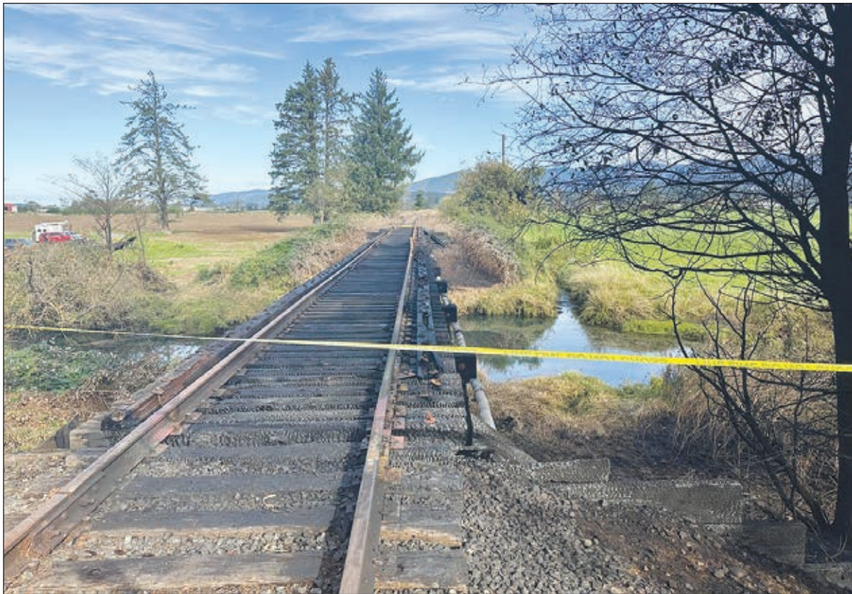
Photo courtesy of Tillamook County Sheriff's Office According to the Tillamook County Sheriff's office, a recent fire on Railroad Bridge near the end of Hadley Road is under investigation.
