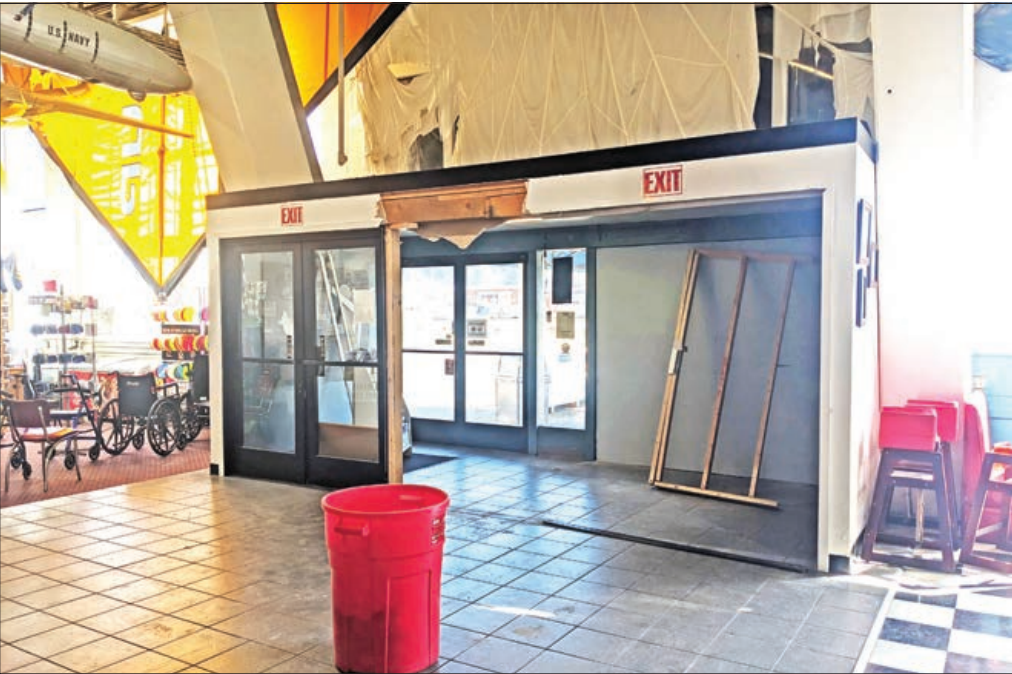
The temporary solution installed by the air museum that allowed them to reopen to guests by October 10. PHOTOS COURTESY OF THE TILLAMOOK AIR MUSEUM AND TILLAMOOK SHERIFF'S DEPARTMENT.
