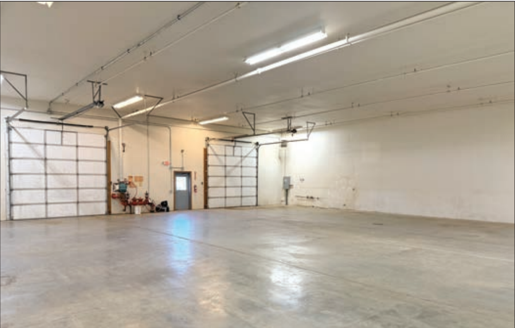
The building’s garage would require significant upgrades to qualify for a change of occupancy and serve as office space.
