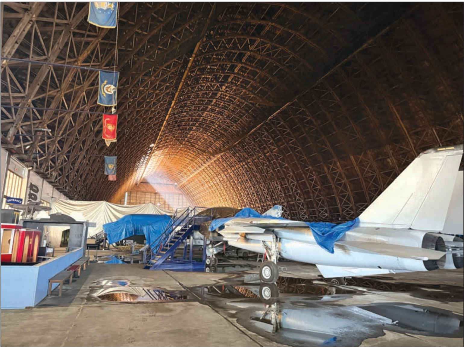
Planes from the Tillamook Air Museum’s collection sit under tarps as the sun pours in through the 200-foot hole at Hangar B’s south end.
