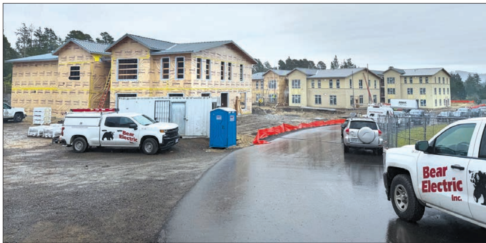
The Spruce Point apartment complex in Manzanita was a hive of work in mid-March, with many tradesmen on site.
