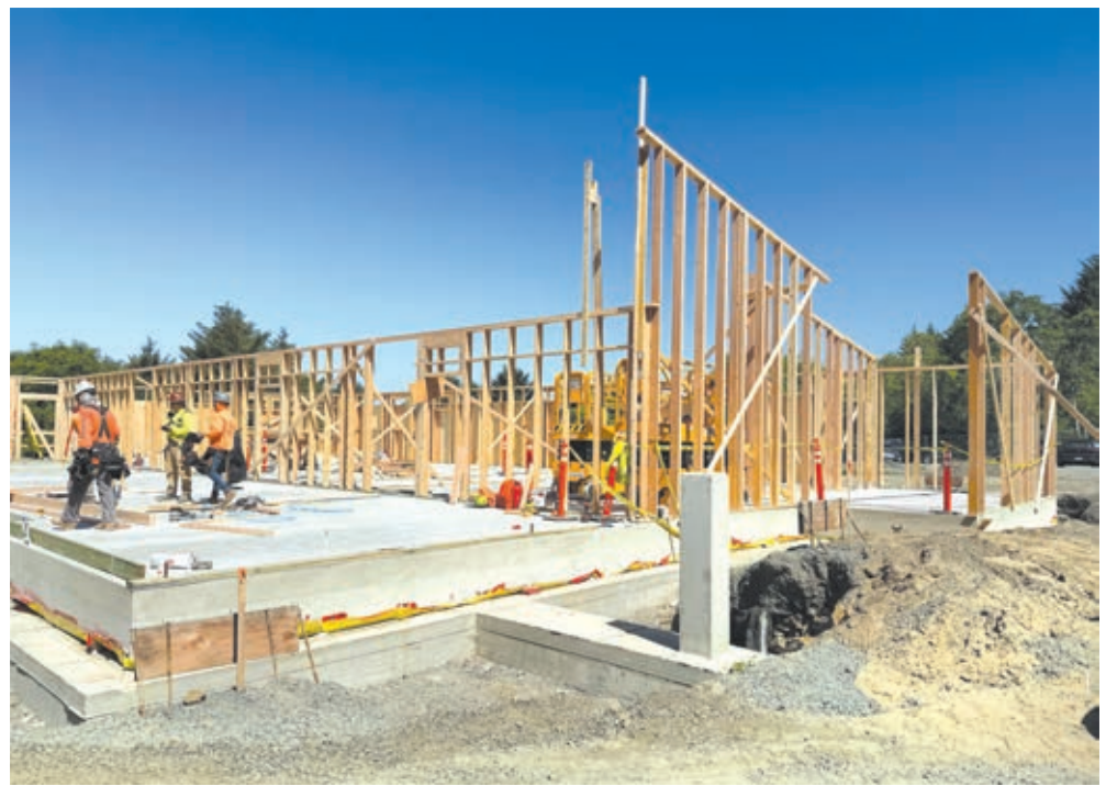
Work underway on the south, public-facing side of the new police department.
