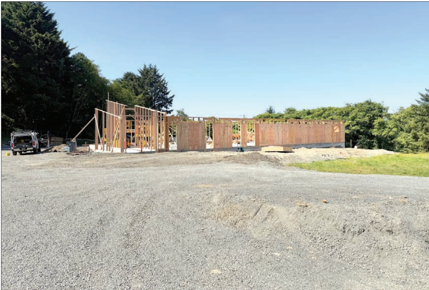
The police station project was taking shape in July as crews erected exterior walls.
