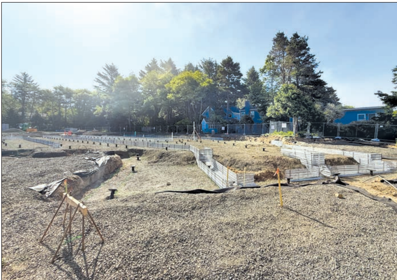
Helical piers had been driven and some forms installed at the police station as a rebar delivery was awaited to complete form installation.
