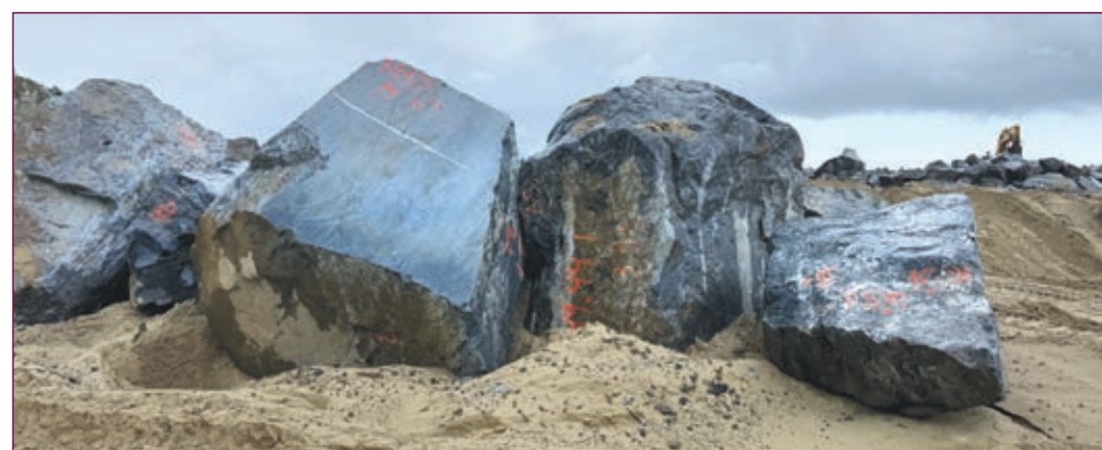
Some of the heaviest stones that will be used in the project, with the one second from left weighing over 49 tons.
