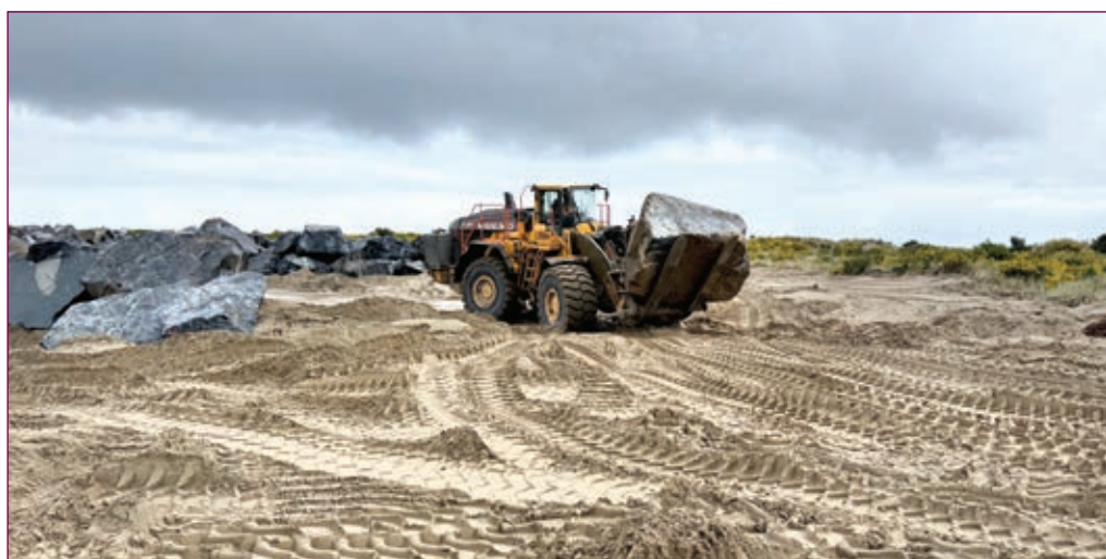
A front-end loader moving a massive rock at the staging area at the base of the jetty.
