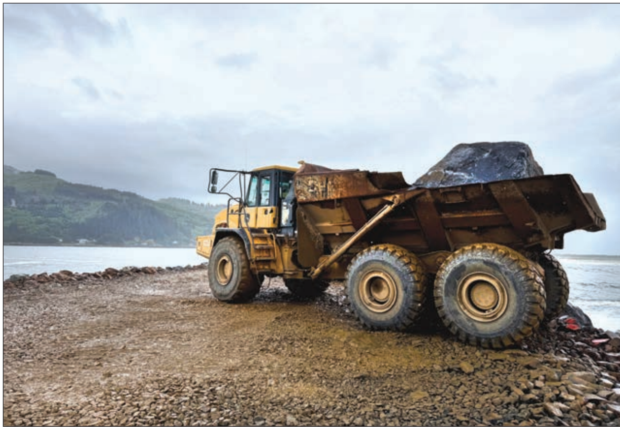
A rock truck maneuvers into position to reverse down the final section of the jetty's trunk to deliver a stone to the placement team at the head.
