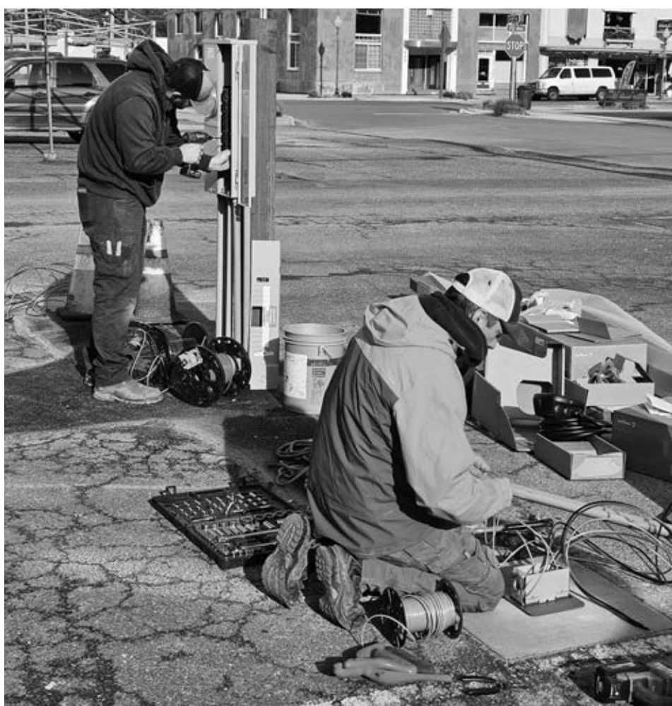
A look at the early days of installation back in December, 2025. The process took nine months, from contracting to completion.
