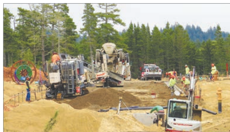
Work on the Cannery Station project has become more visible in recent weeks, with a roadbed, utilities and hydrants being constructed near Highway 101. Tony Reed photo.
