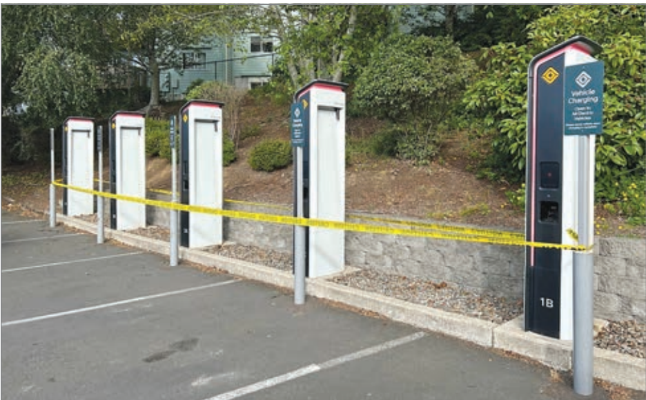
The investigation centered on electrical vehicle charging equipment at the Lincoln City Outlet Mall. (Courtesy photo)
