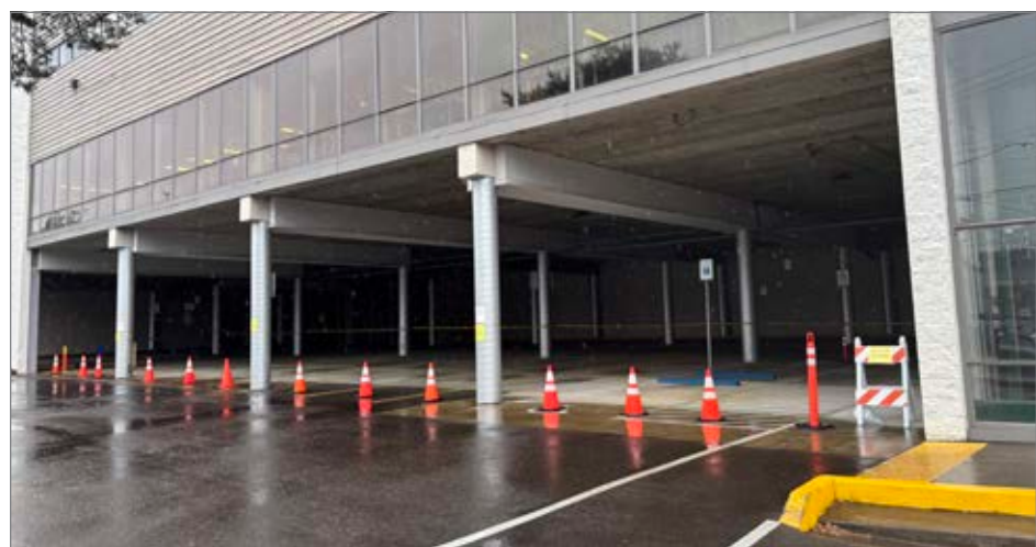
This area of Lincoln Square is closed off due to needed repairs on the fire suppression system that hangs above the parking area at ground level. (Courtesy photo)
