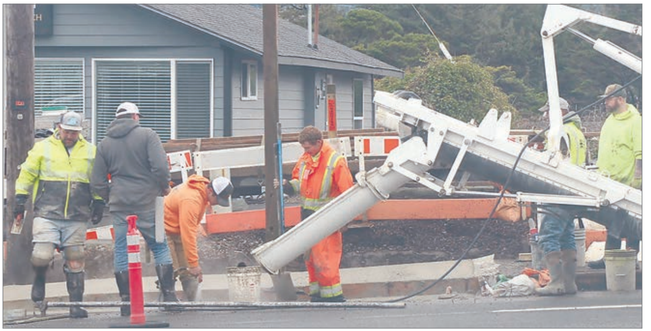
ODOT crews have been working to improve the curb ramps in Lincoln City. (Jeremy C. Ruark / Lincoln County Leader)
