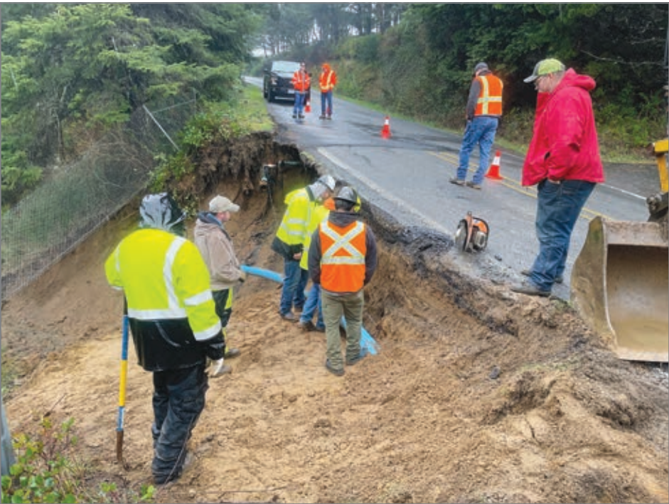
More than a hundred homes were without water last week when a landslide took out a water main on Northeast Beverly Drive north of Newport during the early morning hours of Feb. 28. Work crews were on scene the following morning to make repairs. (Photo by Steve Card)
