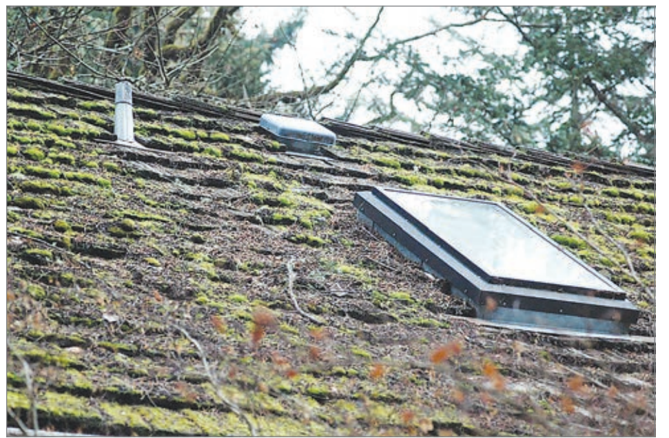
Moss on roofs in the Pacific Northwest is inevitable, but left untreated, it can cause damage that can lead to expensive repairs and replacements. (Courtesy photo)
