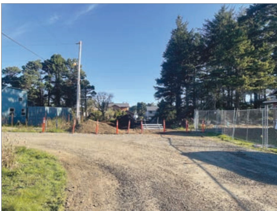
Northwest Biggs Street in Newport currently stops at 59th Street, but as part of the plan to create a drug treatment facility in that area, Biggs is being extended north to 60th Street. Work to clear that area for the street extension was started last week. (Photo by Steve Card)
