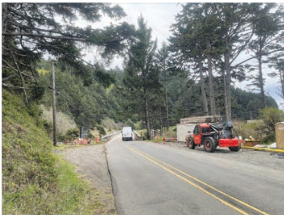
Restoration work is underway on the historic Rocky Creek Bridge, also known as the Ben Jones Bridge, located near the north end of Otter Crest Loop. The bridge was built in 1927. According to a project summary on the Oregon Department of Transportation website, "We're replacing the system that helps prevent the metal from rusting. This is known as cathodic protection. During construction, it'll look like we're painting the bridge." There will be some traffic impacts while work is underway. (Photo by Steve Card)
