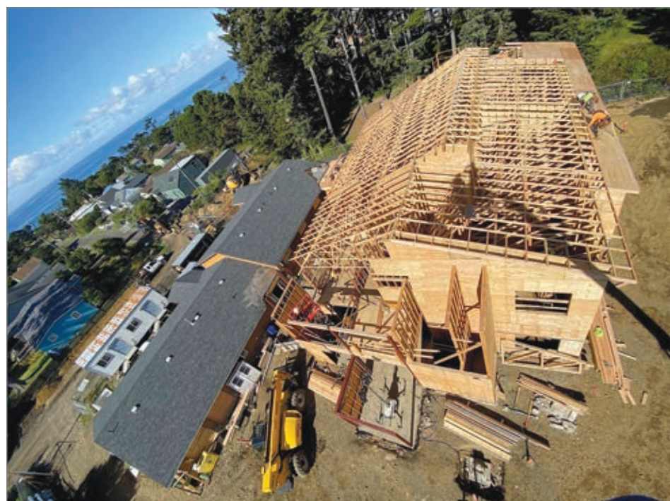
Work is continuing on the construction of the future Samaritan Treatment and Recovery Services (STARS) adult residential and outpatient facility in north Newport. The 8,300-square-foot treatment center will have 16 inpatient beds to serve adults ages 18 and older who are experiencing substance use disorder. (Courtesy photos)
