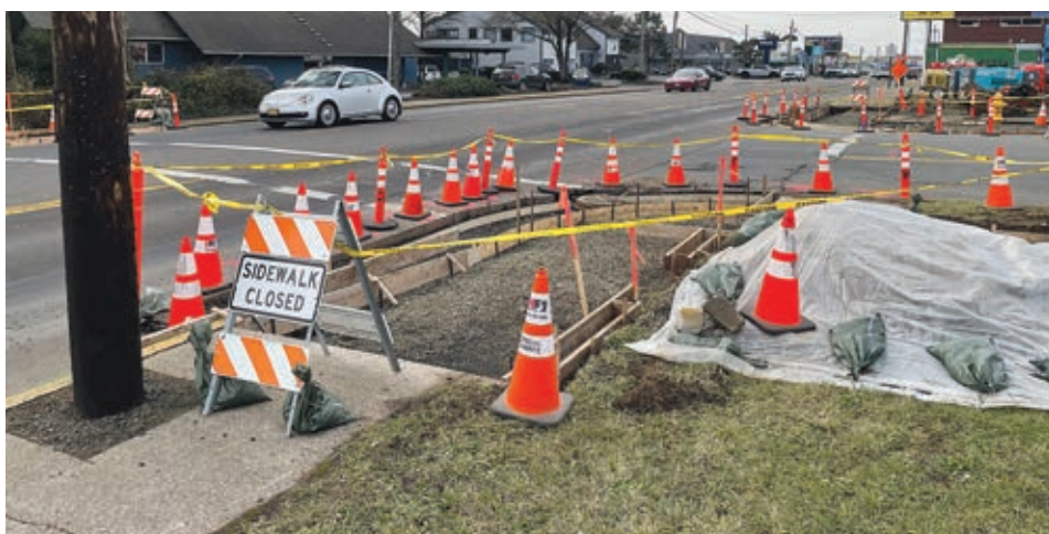
Work is underway to create a safer pedestrian crossing at the intersection of Highway 20 and Eads Street in Newport. The project will include flashing yellow beacons that can be activated by people who are trying to cross the highway. (Photo by Steve Card)
