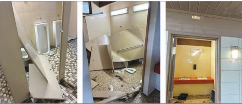
“As you can see the damage is extensive,” OSP Communications Manager Lauren Wistis said. (Courtesy photo)
