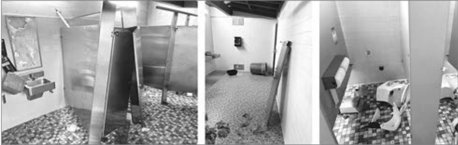
The damage ranges from the removal of paper towel dispensers to the destruction and removal of fixtures and other items from inside the facilities. (Courtesy photo)
