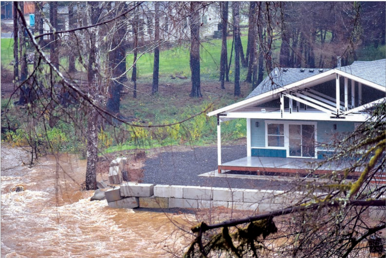
A wall made from concrete blocks collapses into a flooded waterway near Otis in November 2021, when the area saw around 8 inches of rain over a three-day period. (File photo)
