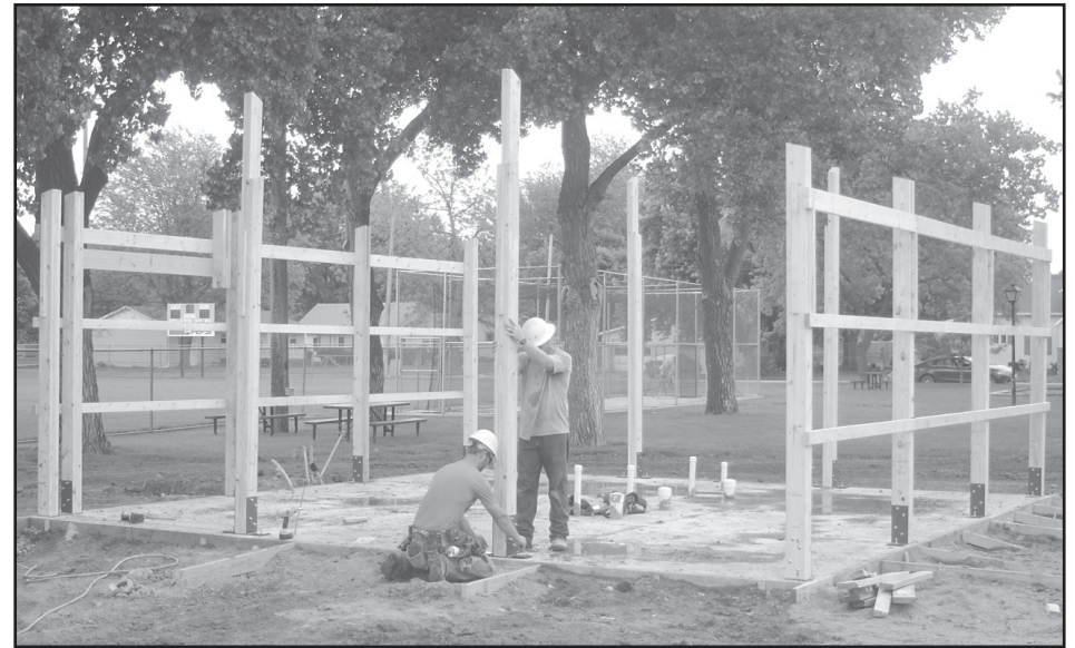
2016 — Morton Buildings of Kearney works on framing the new building at Jaycee Park that will house a concession stand, restrooms and storage for the park.
