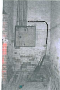
Original electric panel
