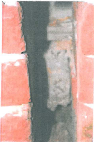
Joist bottom deterioration
