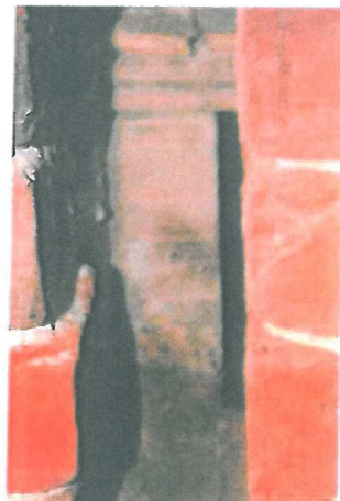
Joist side deterioration
