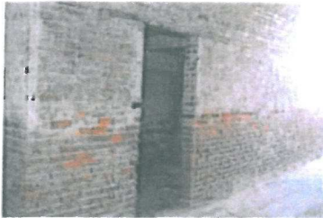
Entry to under stair electric closet
