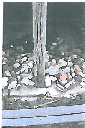
Inadequate base support
