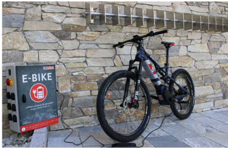
Figure 11 - Electric-assist bicycle charging facility
