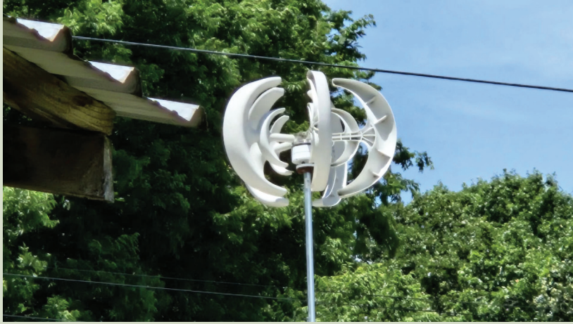
Power generated from nature is the intent of Joe Guthrie, and he powers his living quarters and charging station with wind and solar power.
