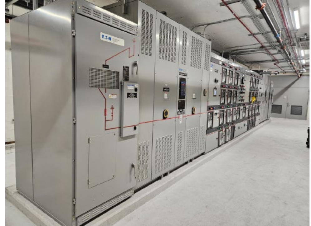
Completed clinical wing substation as an example
