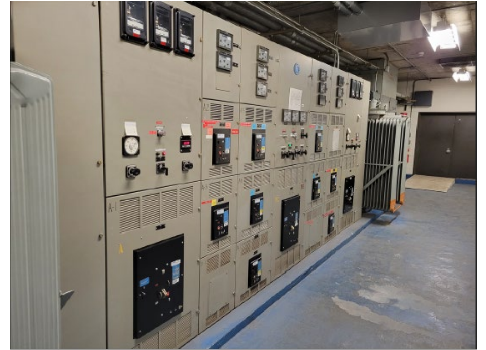
Existing substation to be replaced
