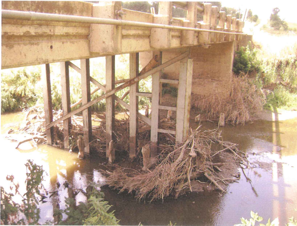
Heavy Debris at Bent 2 – Facing West
