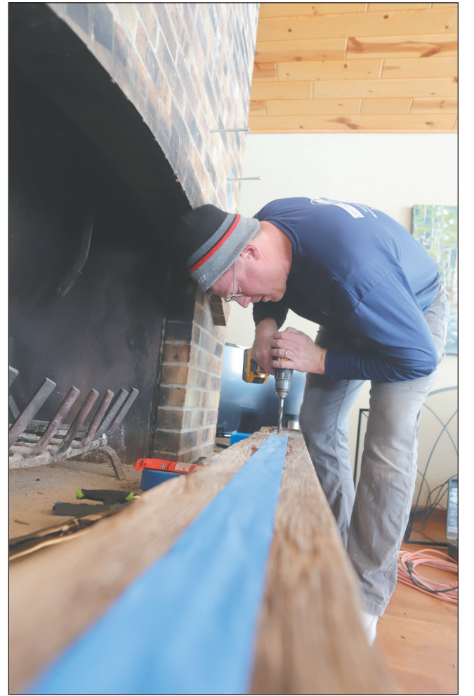
Dann VanDyke drills holes into a piece of wood that the team sourced to be used as a mantel on the fireplace.
