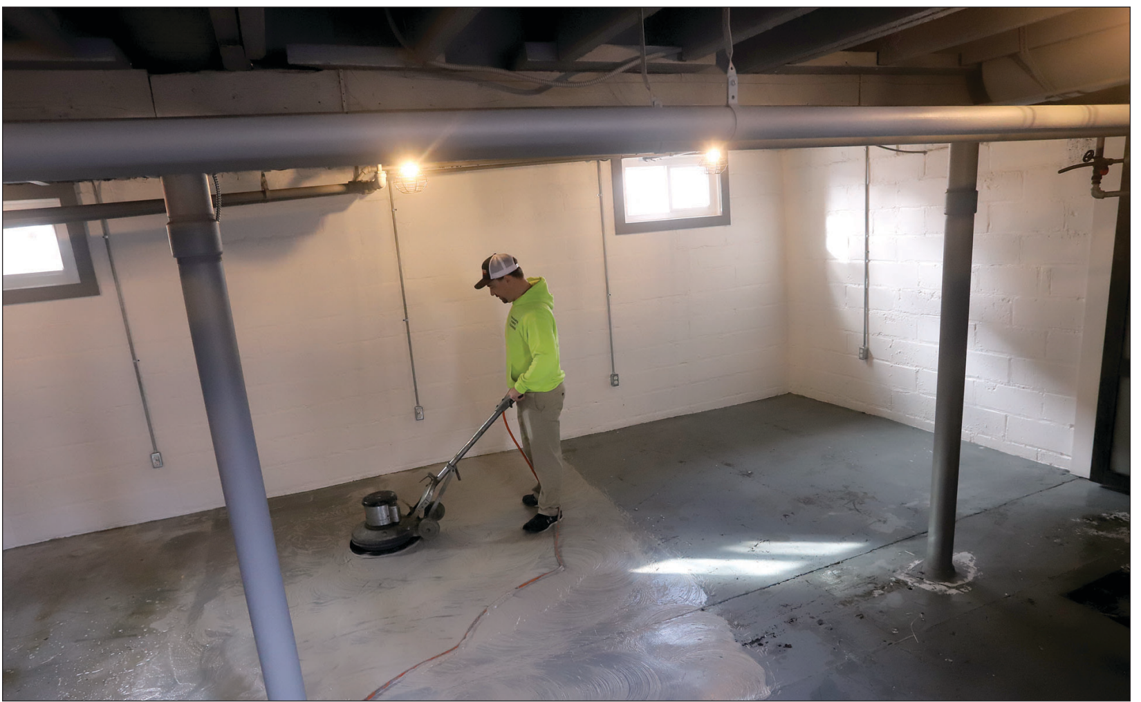
Jason Muralt of ProMaster scrubs the basement floor before it was painted. The basement floor had some areas of grease and dirt that needed to be cleaned before Van Dyke could put down the final coat of paint.
