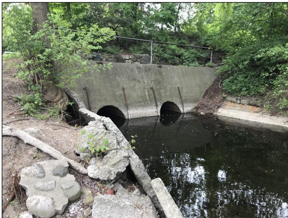
Photograph 55 – Erosion behind auxiliary spillway right wingwall.
