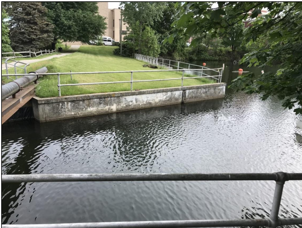
Photograph 4 – Right auxiliary spillway wing wall. Note minor cracking and efflorescence.
