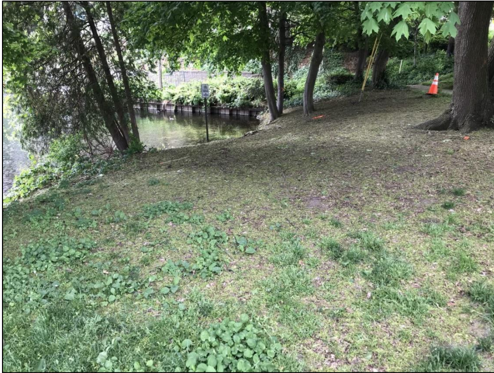
Photograph 1 – Upstream slope at left abutment viewed from auxiliary spillway. Note trees on embankment.
