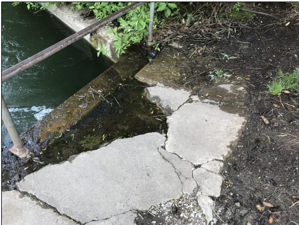
Photograph 39 – Concrete walkway over primary spillway outlet. Note broken concrete and seepage.
