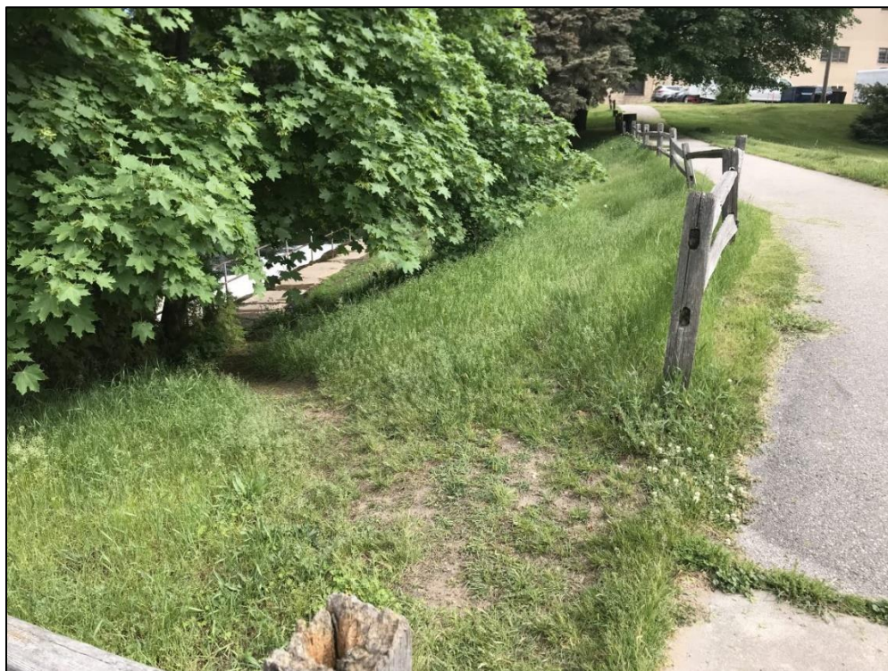
Photograph 15 – Downstream slope of embankment viewed from fish ladder. Note trees and foot traffic erosion.
