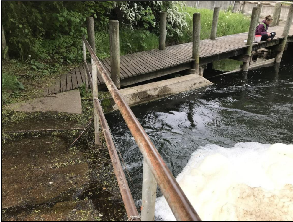
Photograph 43 – Concrete walkway and boardwalk along downstream toe of embankment. Note seepage and broken concrete.
