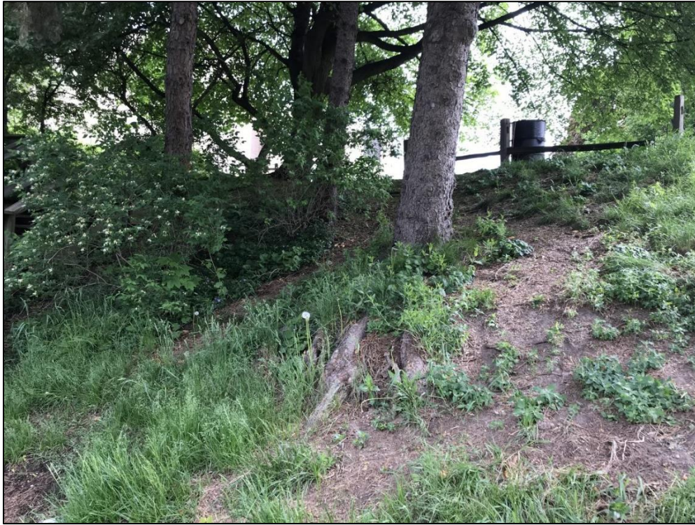
Photograph 38 – Trees and foot traffic erosion on downstream slope near right abutment.
