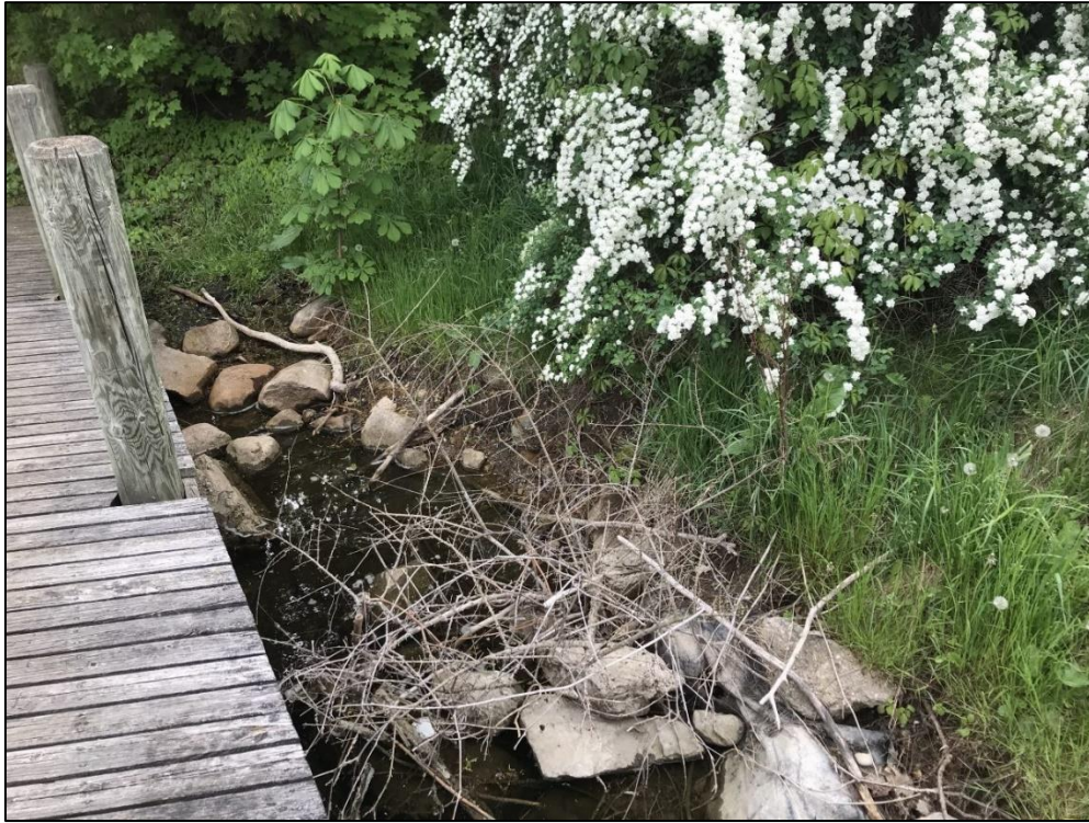
Photograph 47 – Erosion along toe of embankment between primary spillway and fish ladder.
