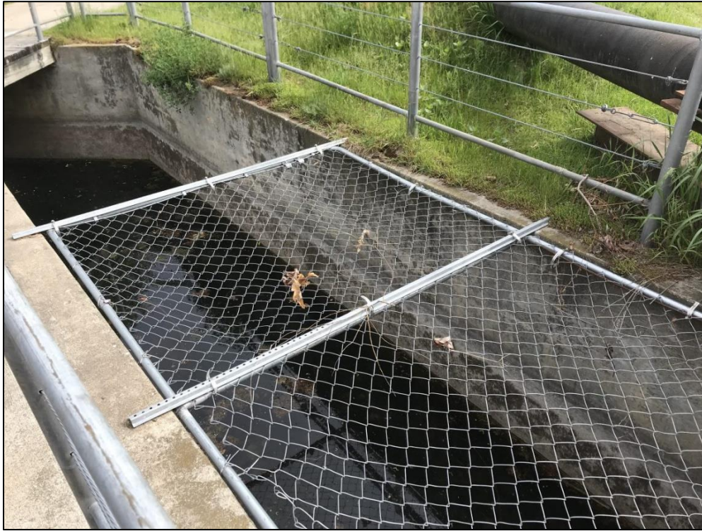
Photograph 11 – Looking downstream at fish ladder from upstream entrance. Note fencing to block fish passage.
