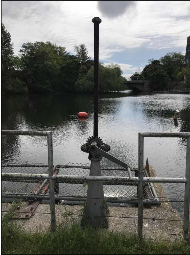
Photograph 23 – Typical gate operator.
