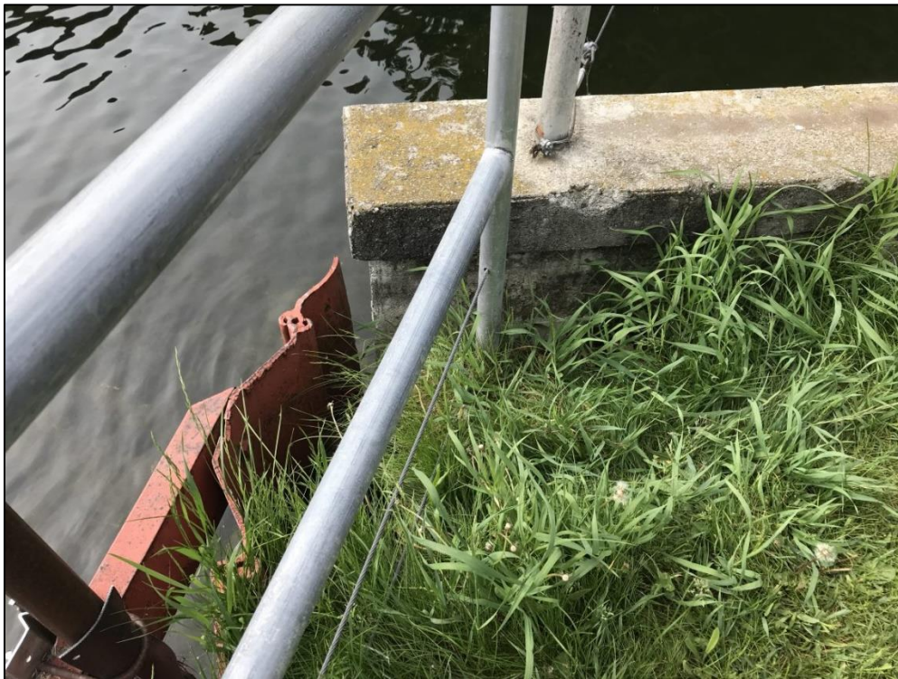
Photograph 20 – Separation between upstream sheet pile and right auxiliary wingwall.
