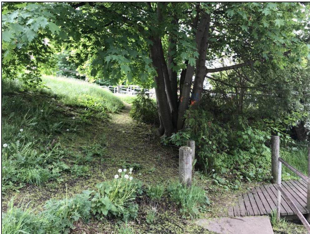
Photograph 44 – Downstream slope of embankment to right of primary spillway. Note foot traffic erosion, trees and vegetation.
