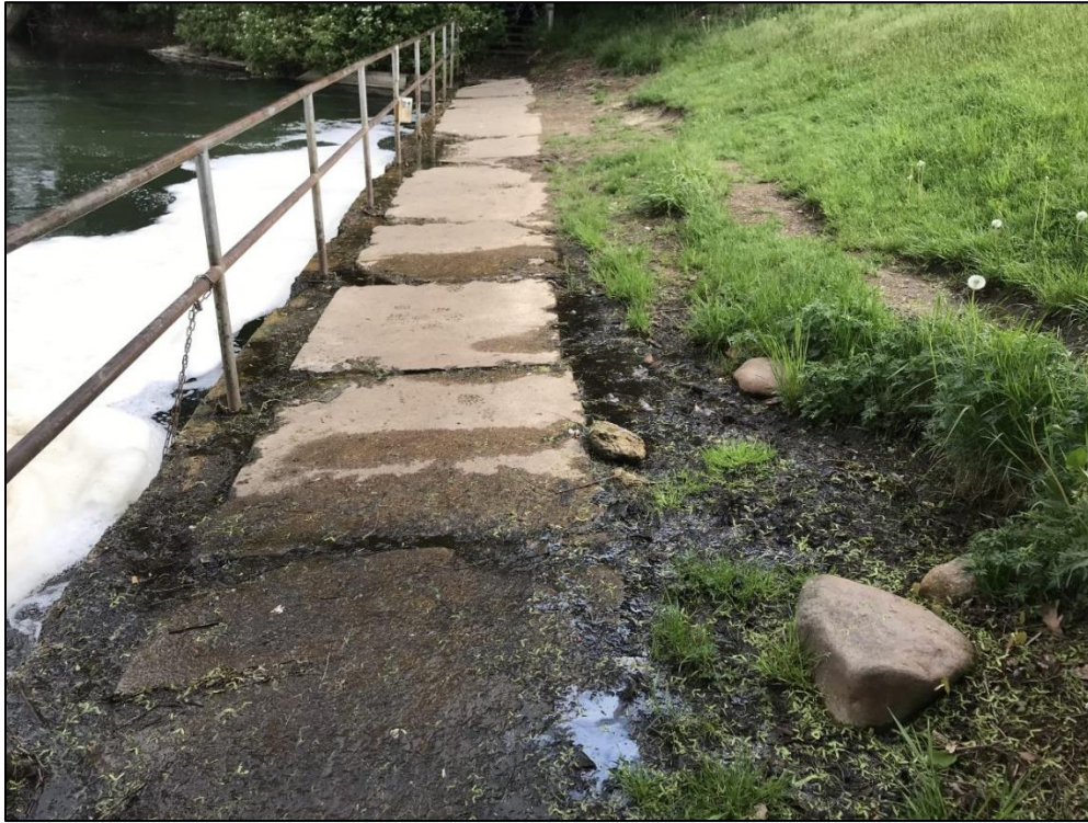
Photograph 45 – Concrete walkway over primary spillway outlet. Note seepage and erosion along toe of embankment.
