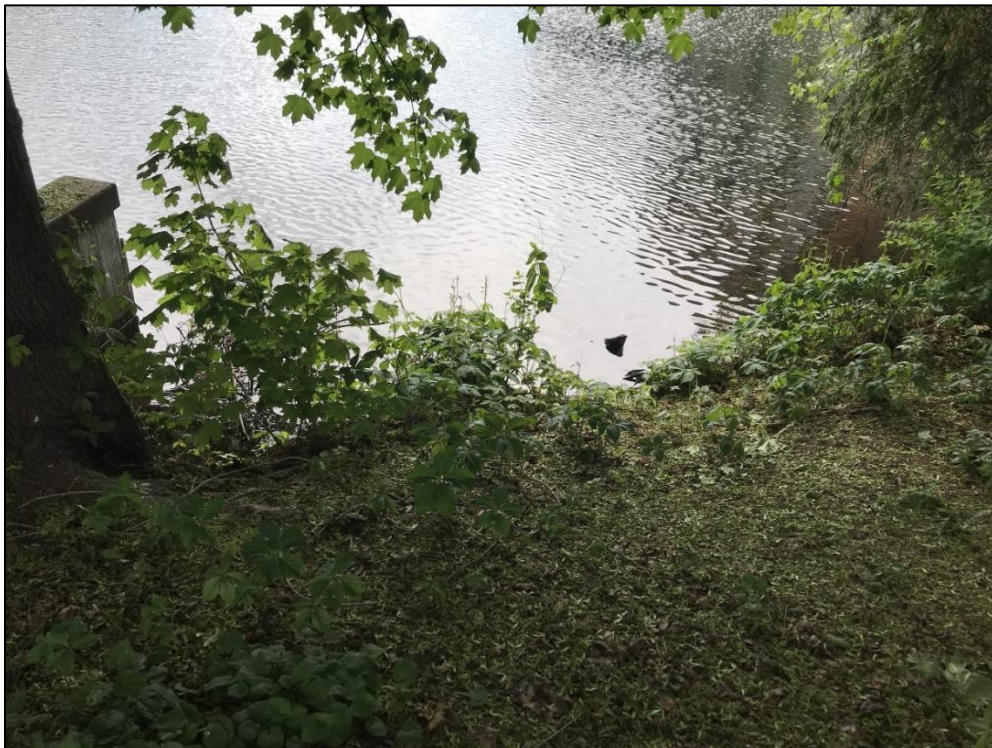
Photograph 2 – Upstream slope left of auxiliary spillway. Note erosion, trees and vegetation.
