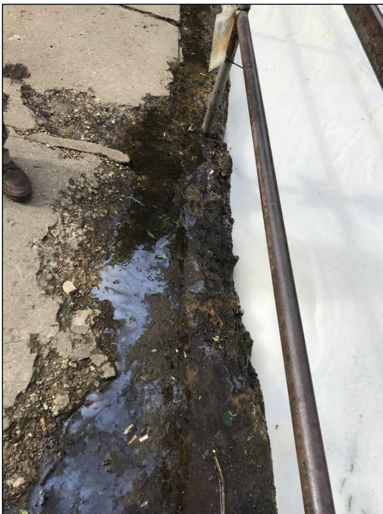
Photograph 42 – Concrete walkway over primary spillway. Note broken concrete and seepage.
