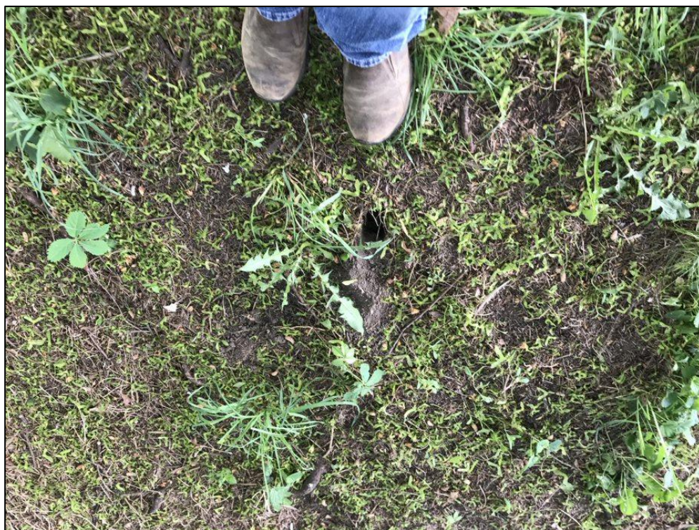
Photograph 37 – Animal burrow on downstream slope near right abutment.
