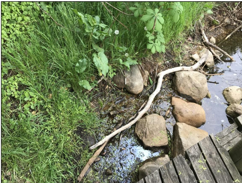
Photograph 48 – Seepage and erosion along toe of embankment between primary spillway and fish ladder.
