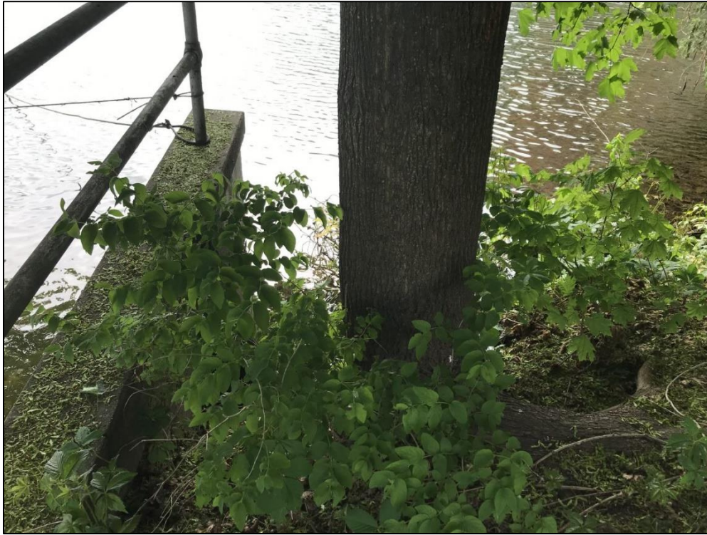
Photograph 3 – Erosion and tree growth adjacent to left upstream auxiliary spillway wing wall.
