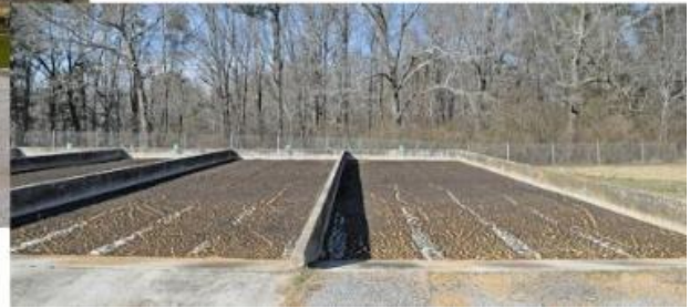
Sludge Drying Bed Facility
