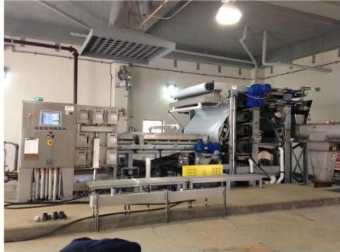
Sludge Belt Filter Press Dewatering
