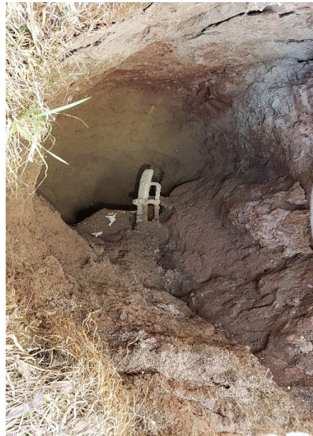
Figure 11. The smaller sinkhole that occurred around 2016 (picture taken in 2020).
