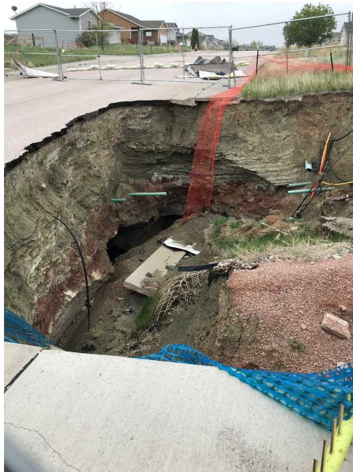
Figure 1. April 27th, 2020 Sinkhole, Hideaway Hills Subdivision, Blackhawk, SD. (picture was taken in May 2021)
