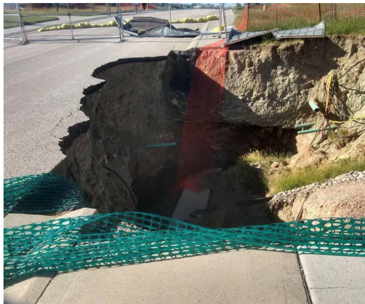
Figure 1. April 27th, 2020 Sinkhole, Hideaway Hills Subdivision, Blackhawk, SD
