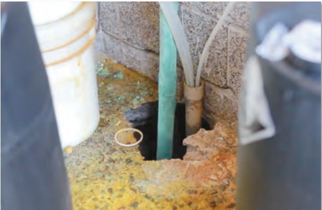
An ISD 12 school in need of repair. The district is offering two planned tours of planned maintenance projects.
