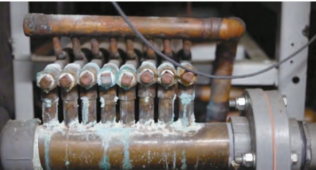
An outdated utilities system. ISD 12’s facilities bond includes a planned $50 million for deferred maintenance projects.
