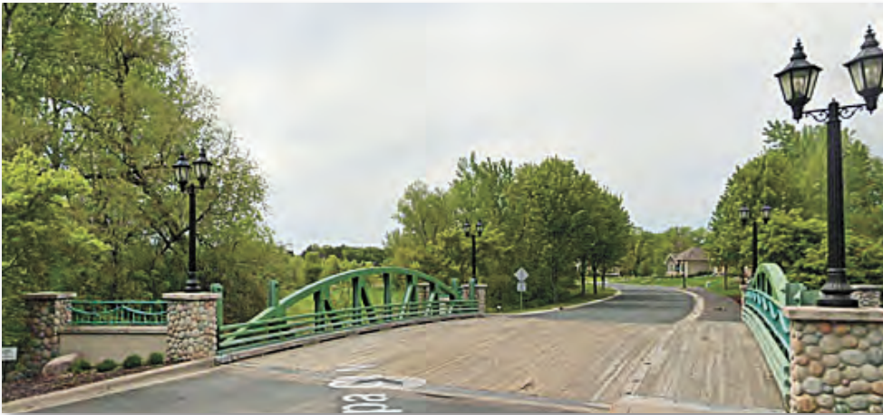
The Fable Hills bridge, which was constructed in 2004, is located over Clearwater Creek and its treated timber deck is starting to fail.
