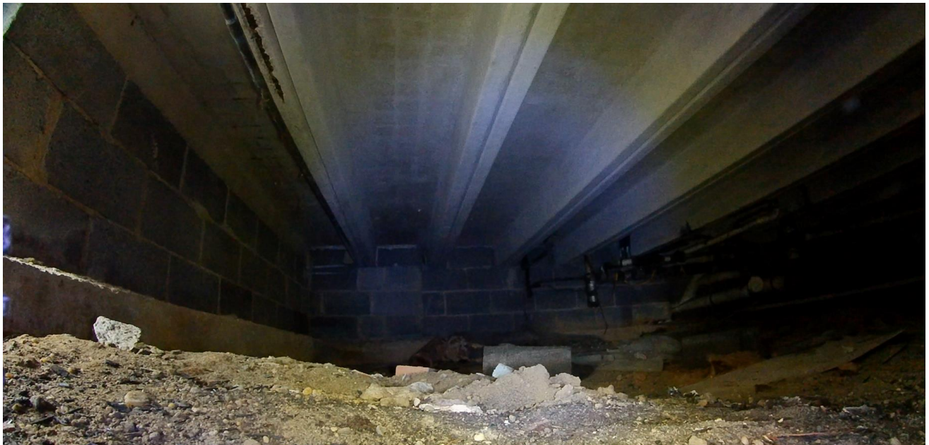
Crawlspace 5 Approximate 1% of Corrosion of reinforcement and concrete spalling in first floor beam
