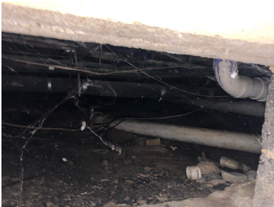
(Crawlspace 1A) Inaccessible Due to Utilities Pipes. Note that concrete and reinforcement corrosion are not in advanced stage
