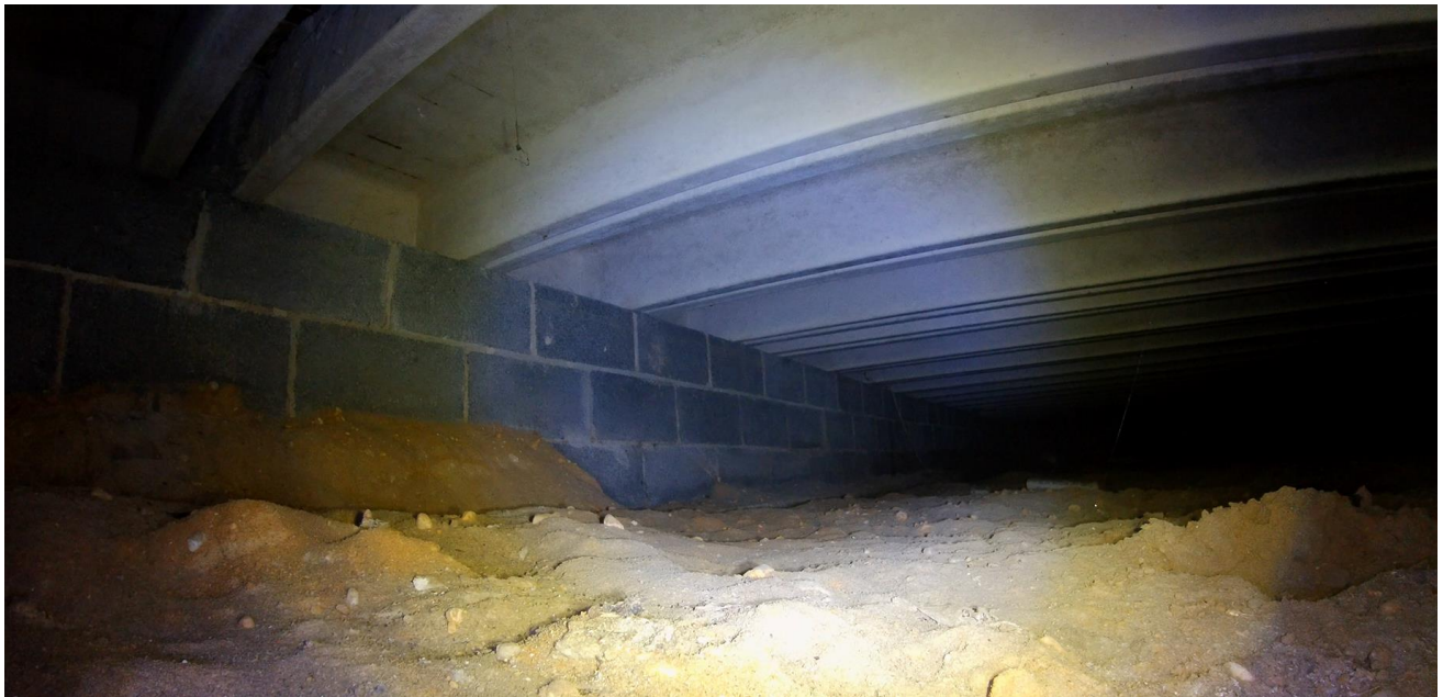
Crawlspace 9 Note that there is a crack in the CMU wall need to be repaired.
