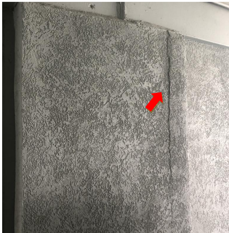
Southwestern side (Units 17 ~ exterior) Note cracks through the walls
