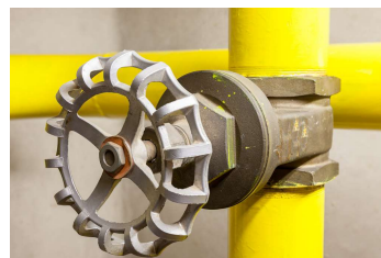
Master shut-off gate valve
