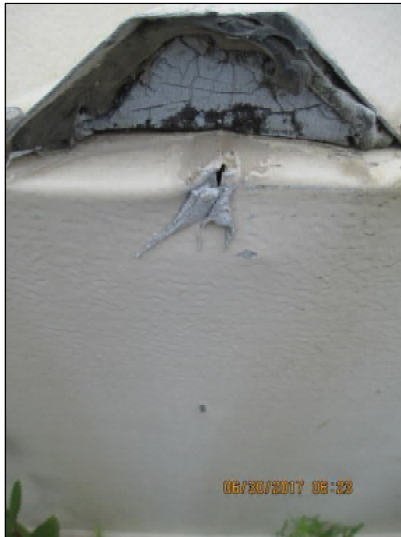
Photograph 13: Repairs are needed at Reservoir 62310.
