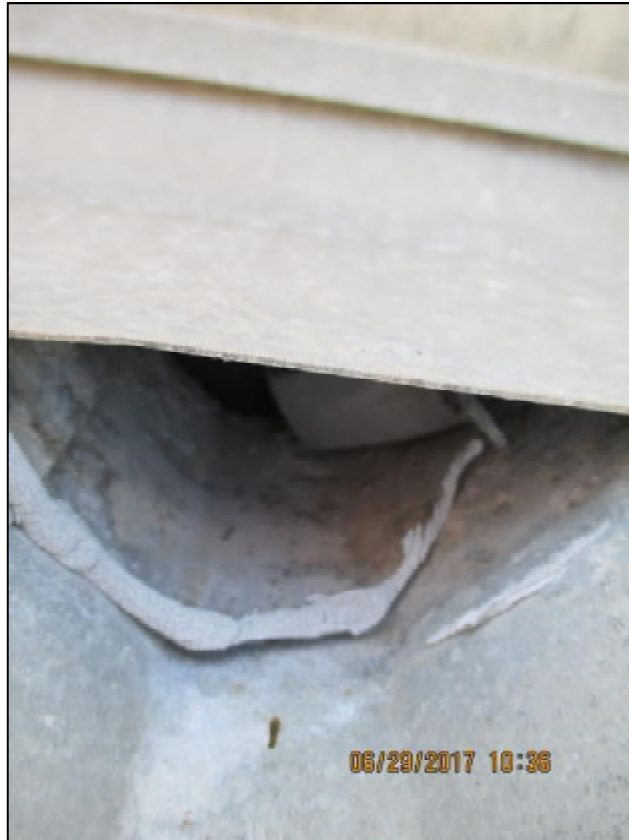
Photograph 5: For Reservoir 51771, some of the divot plugs between the corrugated roof and the vent need repairs.
