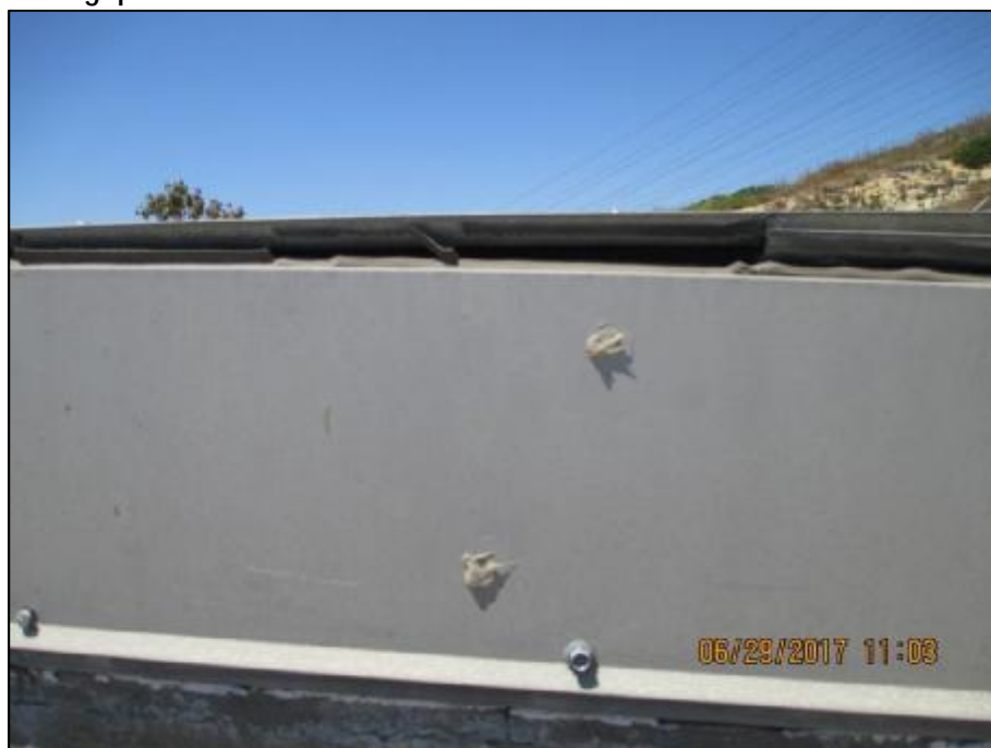
Photograph 12: A gap in between the roof and the wall at Reservoir 51772.
