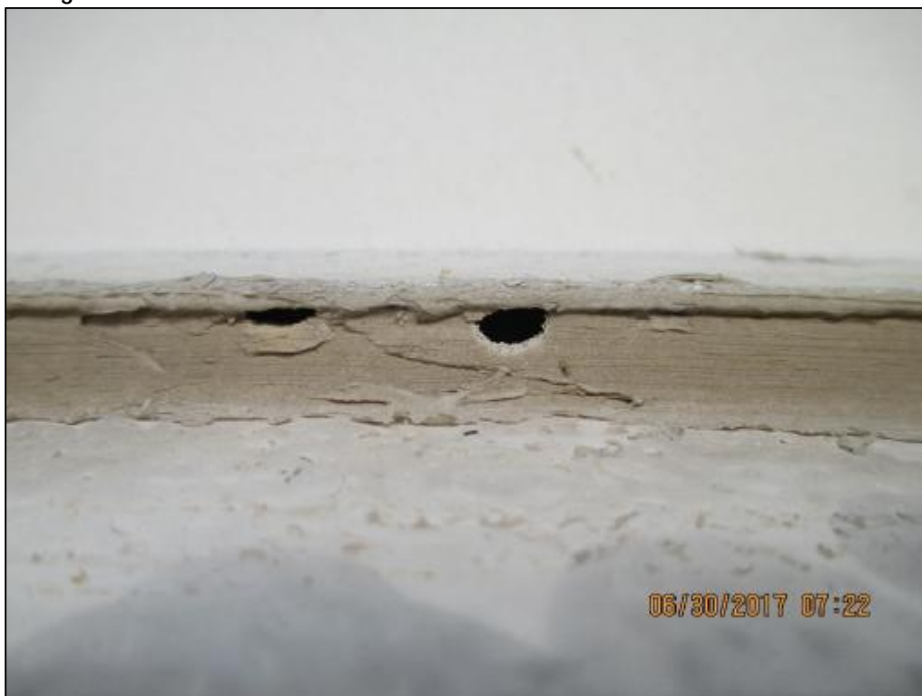
Photograph 20: The sealant between the roof of Reservoir 63210 and the wall had some minor cracks forming.
