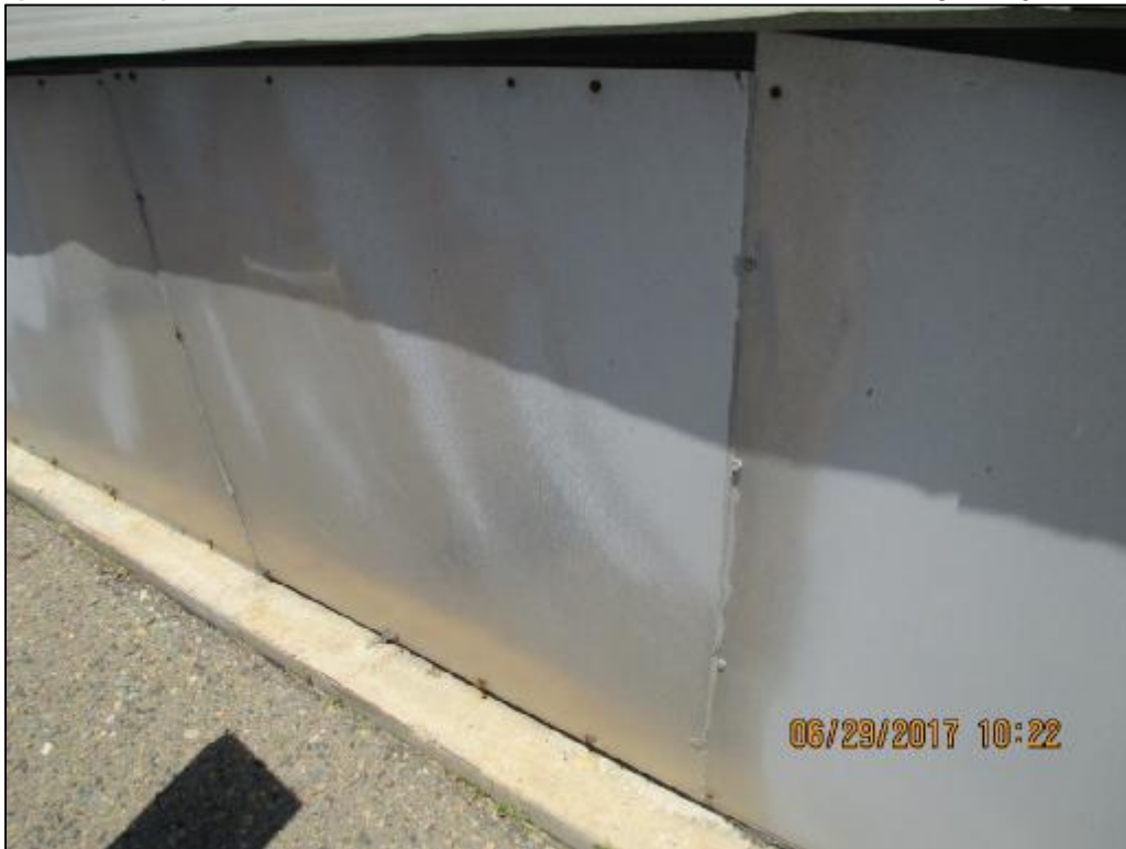
Photograph 3: The panel walls for Reservoir 51770 were loose and missing many bolts.
