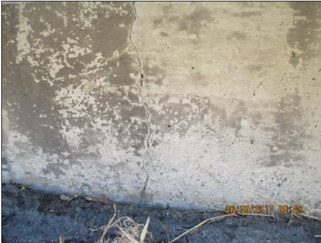
Photograph 25: A crack along the wall of Reservoir 53116
