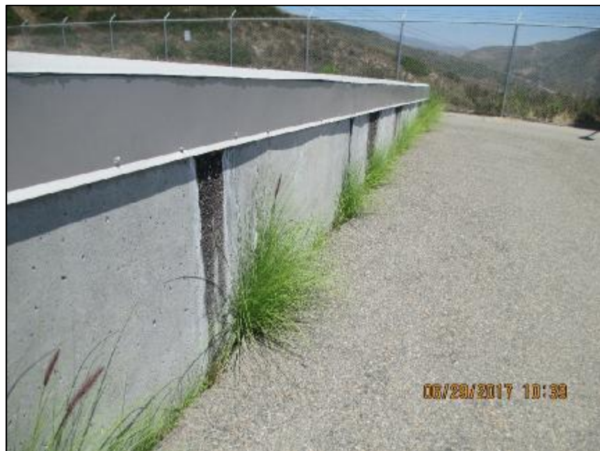
Photograph 6: There was evidence of condensation in Reservoir 51771 leaking along the outside of the concrete walls.
