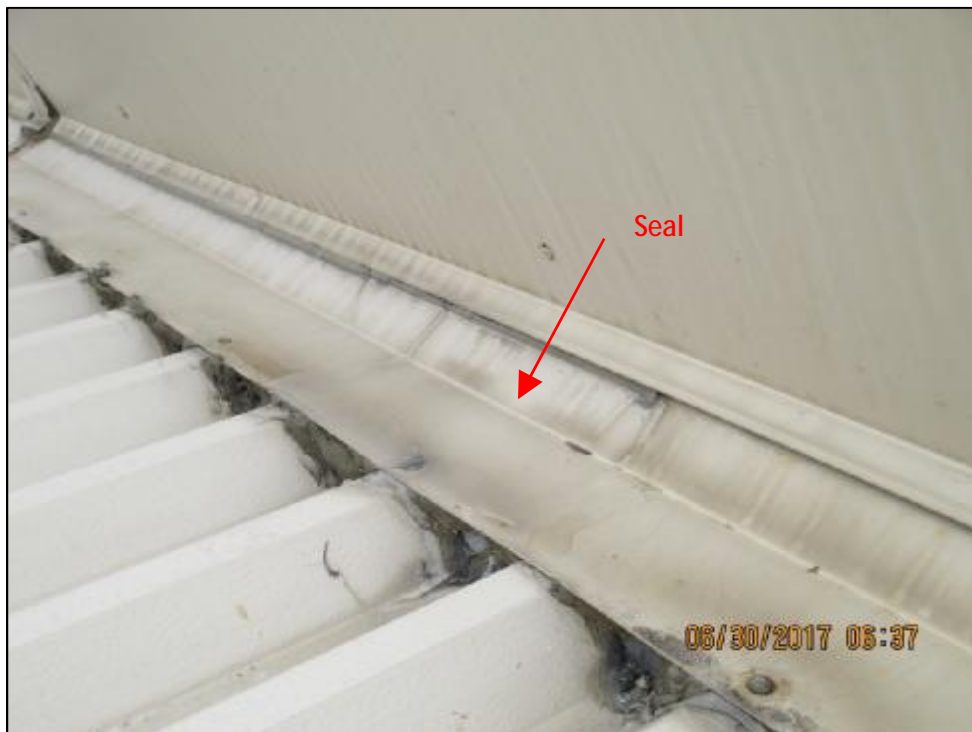
Photograph 14: The upward facing vent had a seal along the base that would prevent rain water from exiting the vent. This may lead to rain accumulation that would enter Reservoir 62310.
