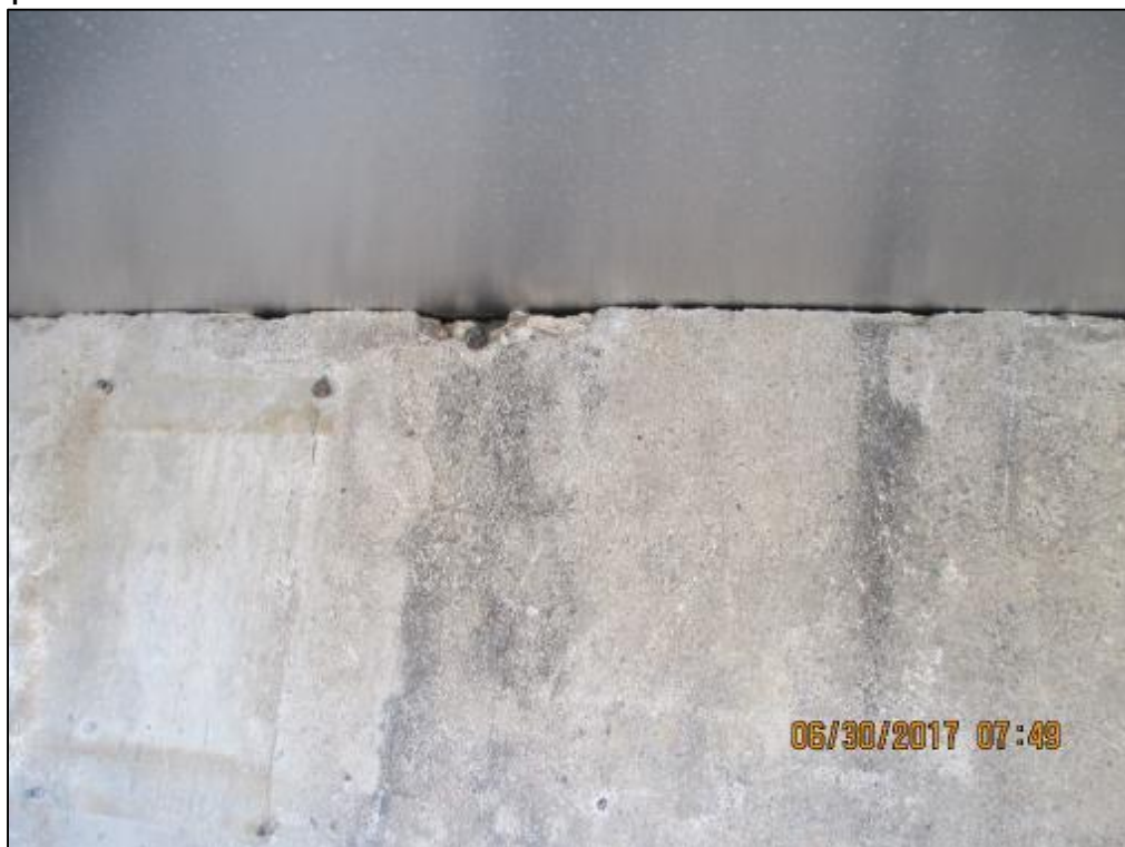
Photograph 22: The concrete roof and the metal roof need a seal at Reservoir 52698.
