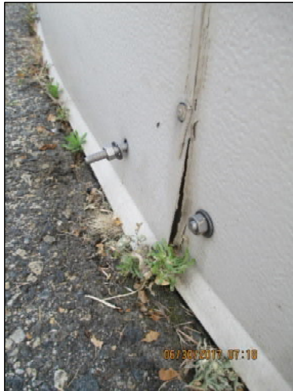
Photograph 17: the paneling at Reservoir 63210 was coming off and needs repairs. Gaps are created by loose siding and holes from loose bolts.
