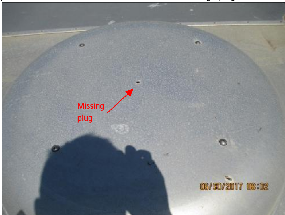
Photograph 23: One of the vents for Reservoir 52698 was missing a plug on the vent roof.
