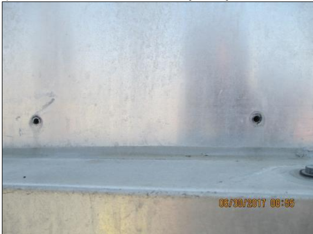
Photograph 26: Reservoir 53116's wall had bolts missing, creating holes in the reservoir.
