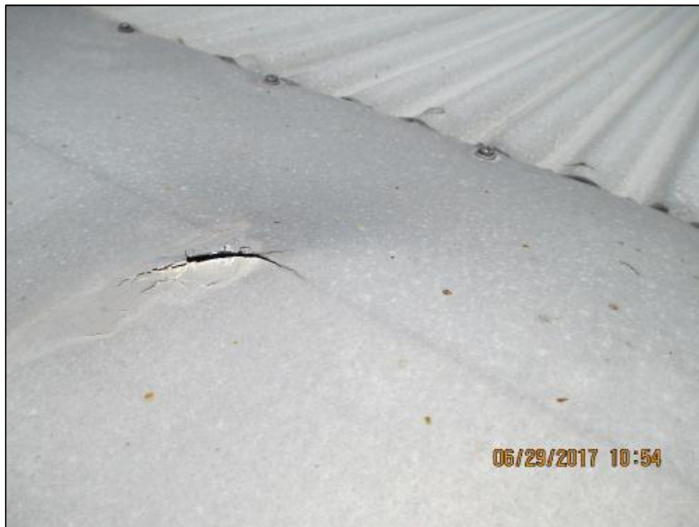
Photograph 10: A crack in the roof of Reservoir 51772.
