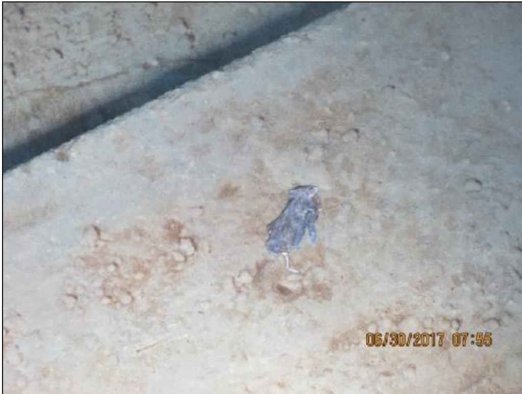
Photograph 21: A dead rodent was found in the finished water of Reservoir 52698.
