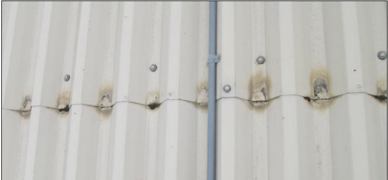
Photograph 15: Reservoir 62310 had moss growing in the seams between the roof panels.
