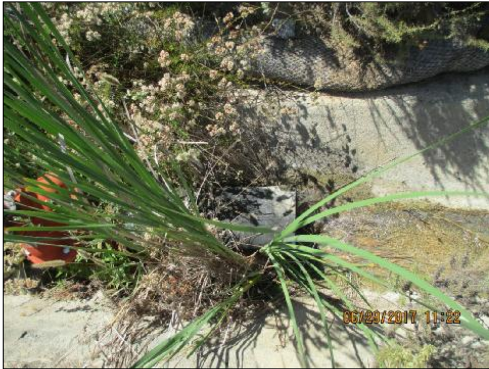
Photograph 7: Reservoir 51771's overflow valve was too close to the ground and surrounded with brush. In addition, the overflow was constantly leaking water.
