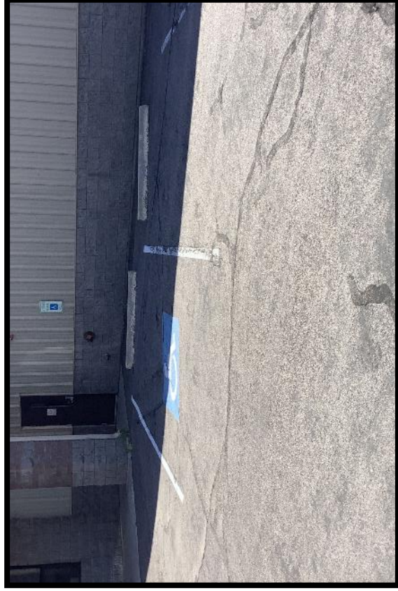
MISSING ACCESS AISLE
