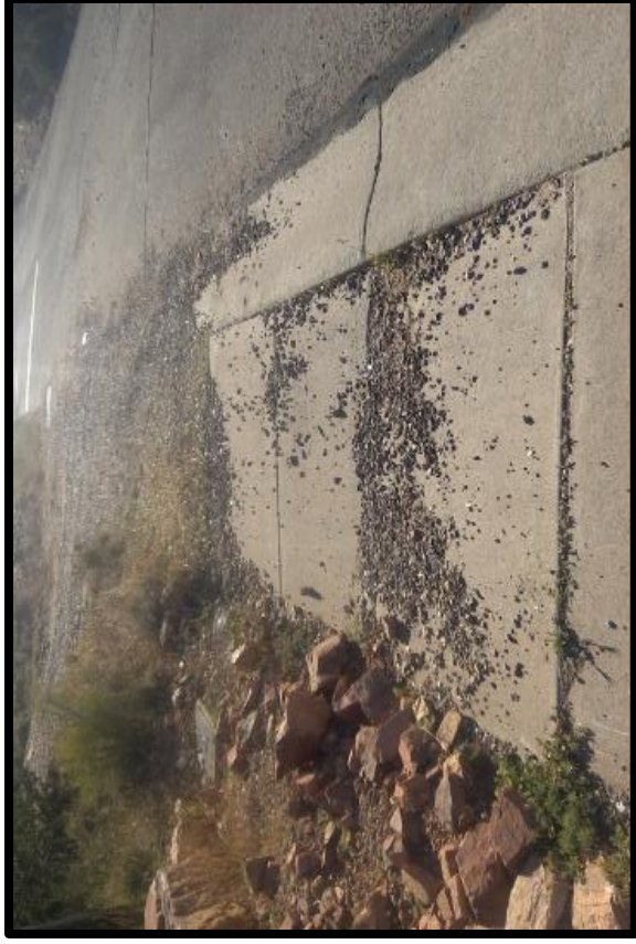
SINKING, CRACKING, AND PONDING
