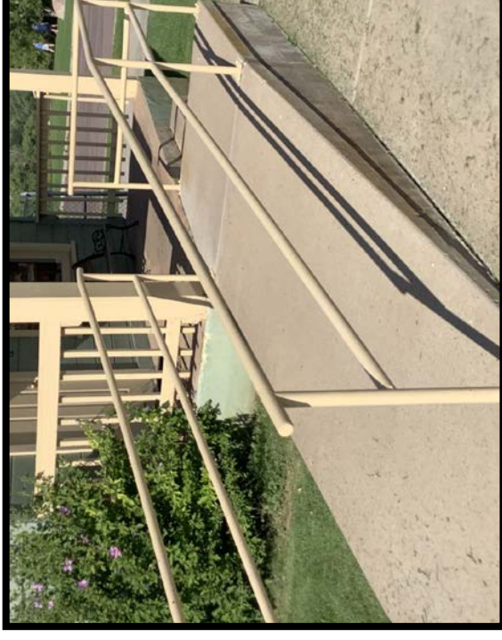
MISSING HANDRAIL EXTENSIONS AND EDGE PROTECTION RIM COUNTRY MOUNTAIN
