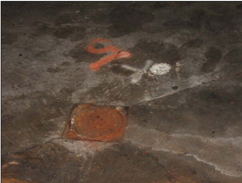
10. Floor drain near B-5 from previous environmental assessment.
