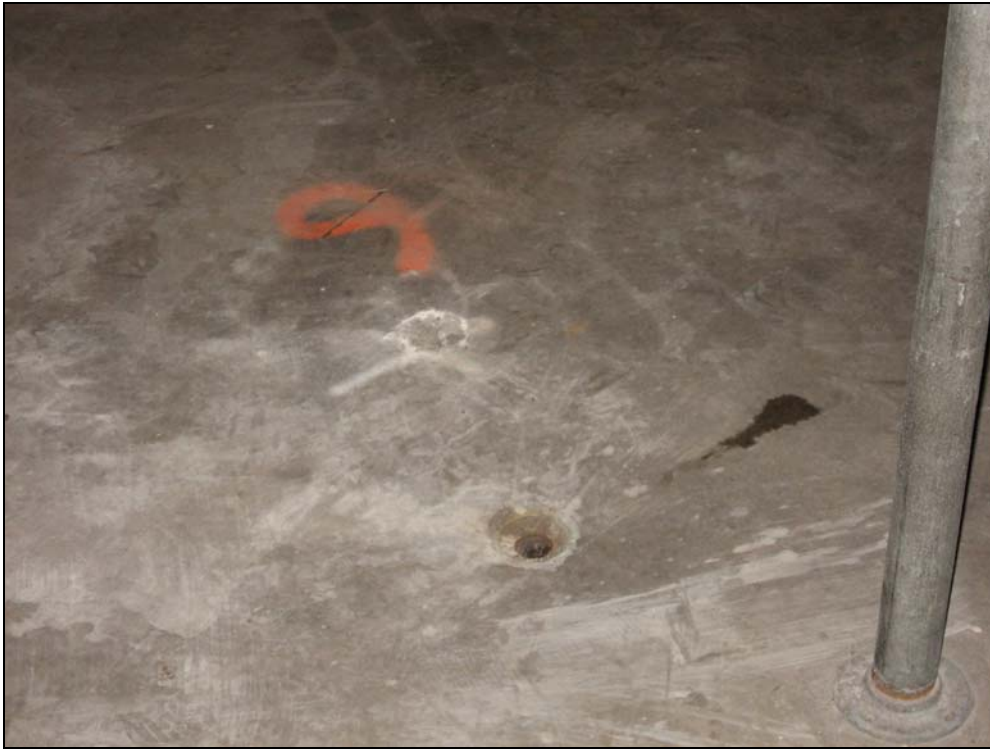
11. Floor drain near B-6 from previous environmental assessment.
