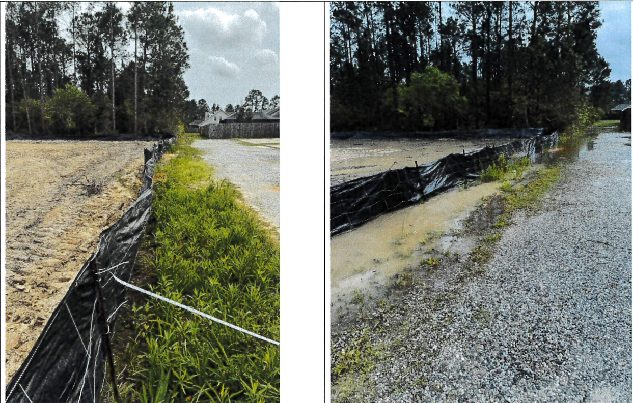
Photo 3&4: Looking South along silt fence (left photo); Looking south along silt fence. The silt fence is essentially in the centerline of the drainage ditch. This does not adhere to/violates Storm Water Pollution Prevention Notes 1, 3, and technically 6. Just after a rain event photo on the right depicting ineffective pollution prevention/sediment load in the ditch.
