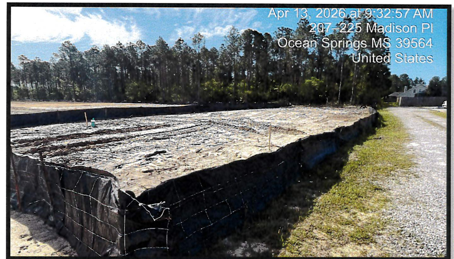
Silt fence will be removed from drainage conveyance and vegetation will be planted to restore impacted area.
