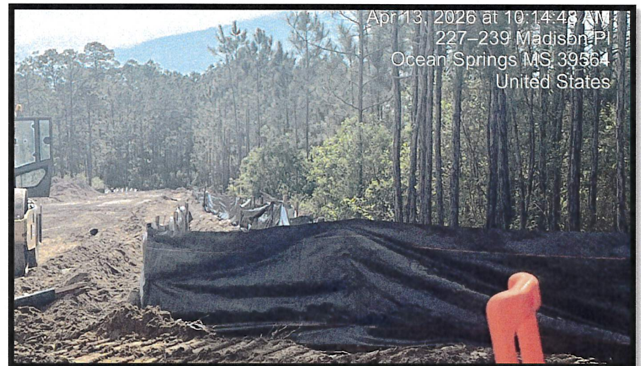
Double row silt fence installed along rear of lots. Piping is currently being installed to allow for stormwater drainage.
