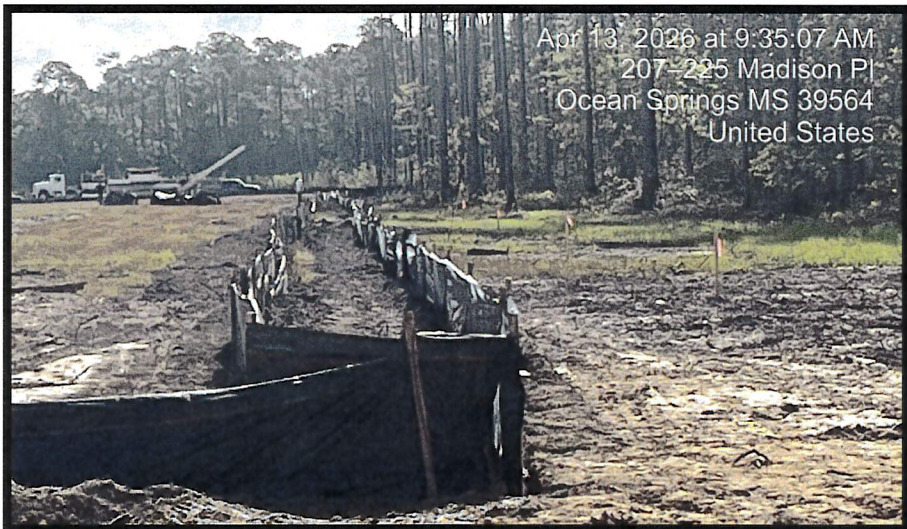
Double row silt fence along rear of lots. Previously impacted area in front of silt fence will be stabilized.
