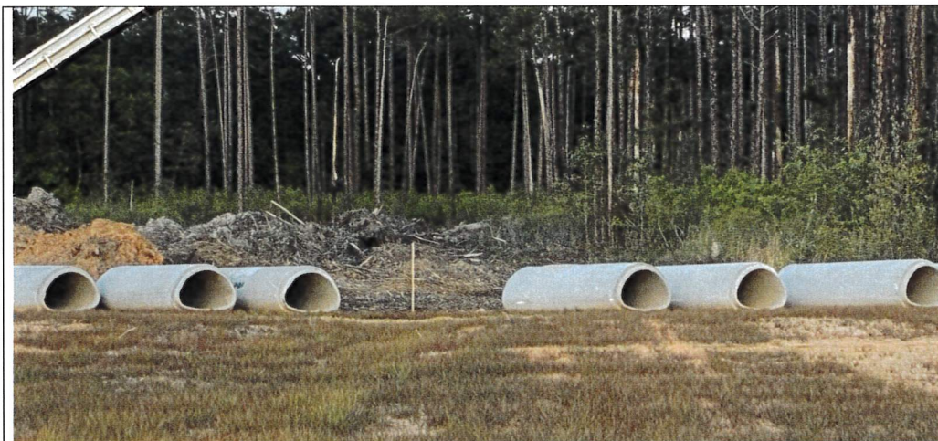
Photo 6: Looking east from Gibson Road, behind proposed lots 31-39; there is no erosion control between the current grading and forested wetlands/conservation easement
