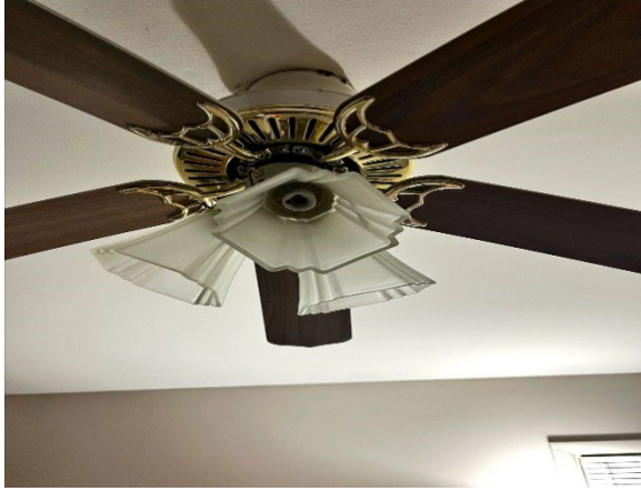
Photograph 7: Light fixture with no lighting
