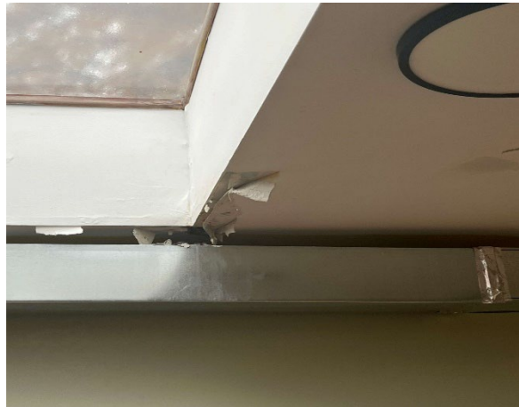
Photograph 6: Peeling paint on ceiling
