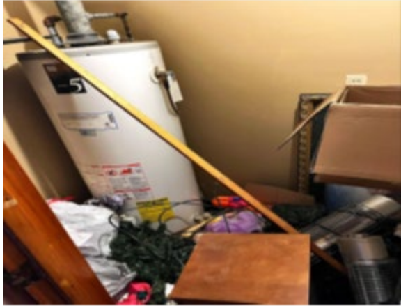
Photograph 11: Debris surrounding water heater containing open flame
