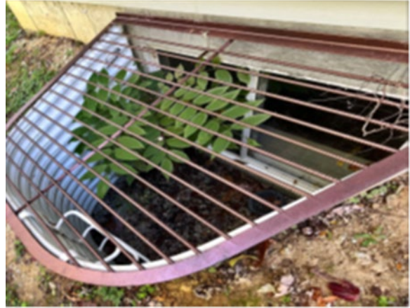
Photograph 12: Heavy grate blocking bedroom emergency exit from basement
