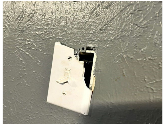
Photograph 16: Broken light switch
