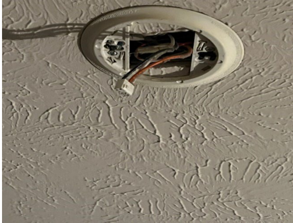
Photograph 17: Missing smoke detector with exposed wiring
