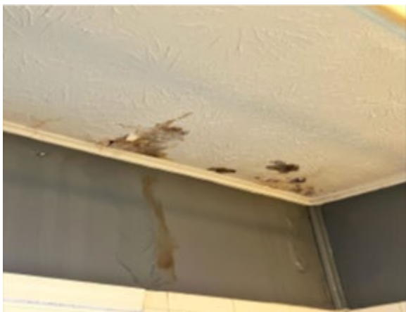
Photograph 1: Water damage and mold on ceiling and wall
